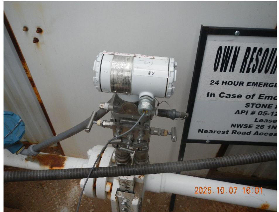
6. Gas meter inside remote meter shed.
