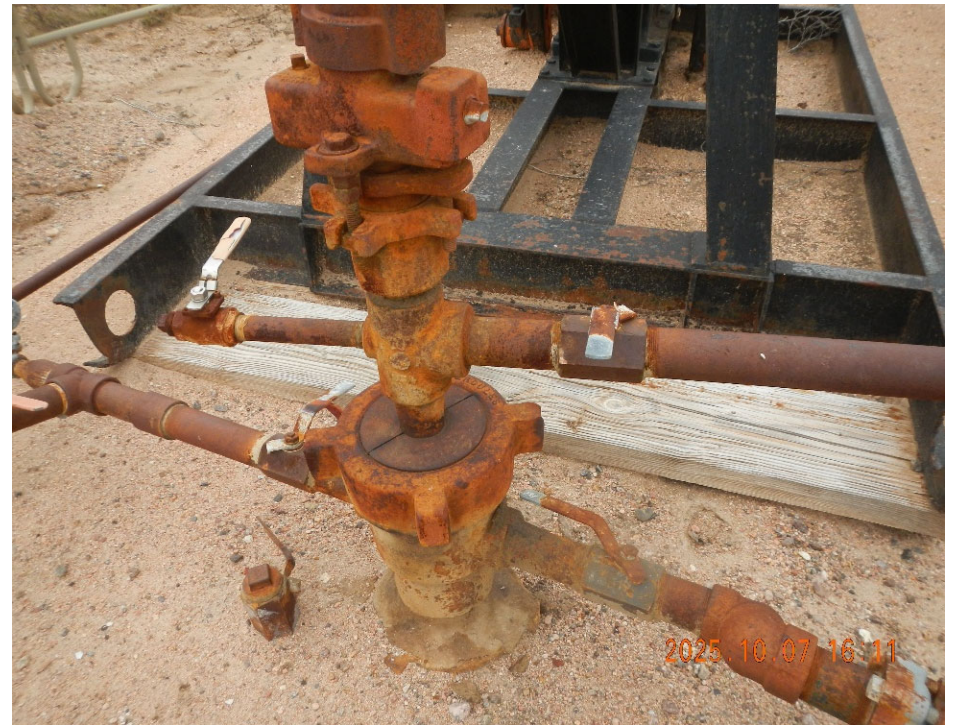
2. View of wellhead.
