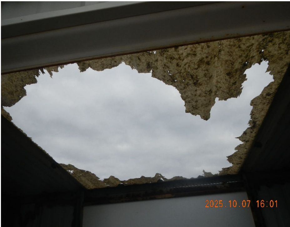
5. Damage to remote Meter Shed roof.
