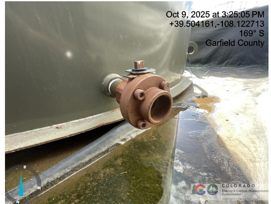
Photo # 5812 Open ended load line
