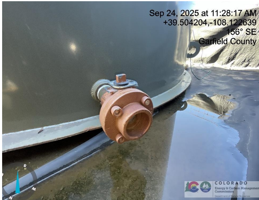
Photo # 2177 From inspection/audit 708907542 conducted on 09/24/2025 - Open ended load line
