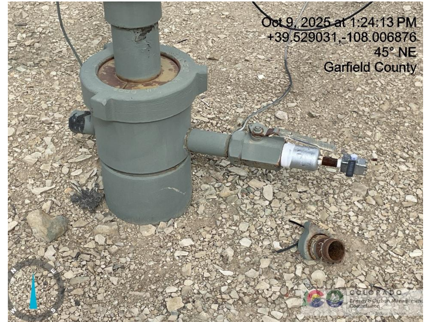
Photo # 5385 Open ended pipe near wellhead/wildlife hazard/available for entry by wildlife
