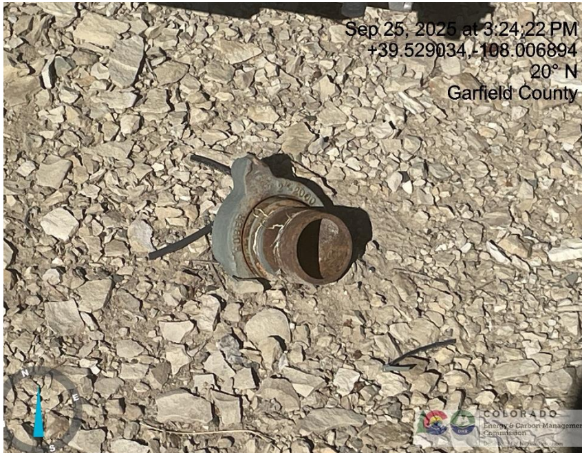
Photo # 3210 From inspection/audit 708907551 conducted on 09/25/2025 Open ended pipe near wellhead/wildlife hazard /available for entry by wildlife
