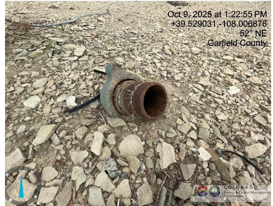
Photo # 5386 Open ended pipe near wellhead/wildlife hazard/available for entry by wildlife
