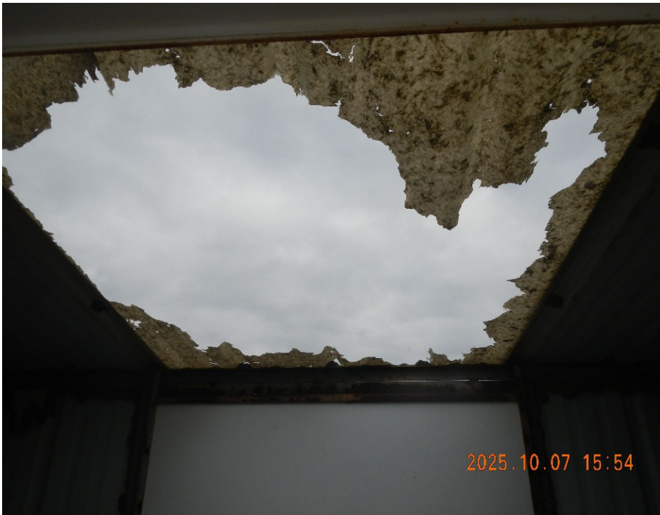
5. Roof damage on Gas Meter Shed.
