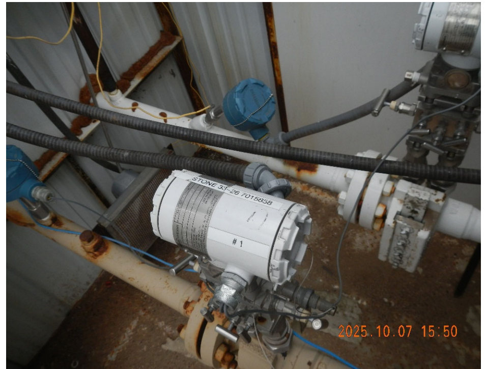
6. Gas meter inside meter shed.
