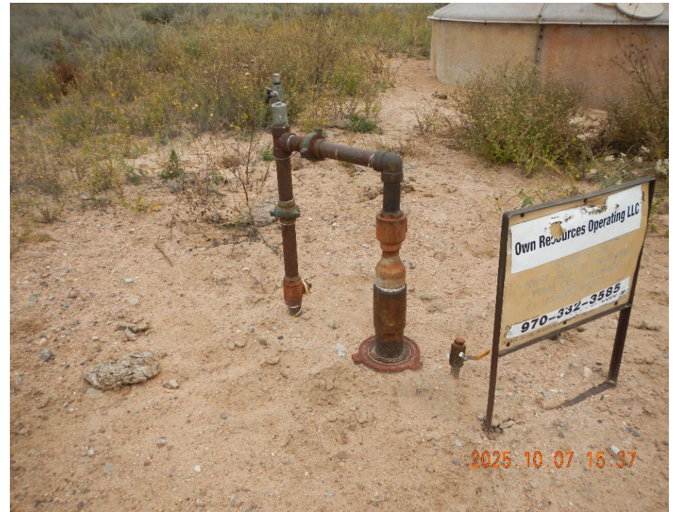
2. View of wellhead.
