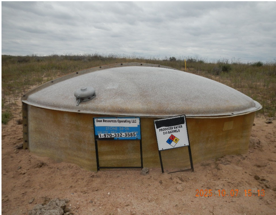
3. View of Production tank at well location.
