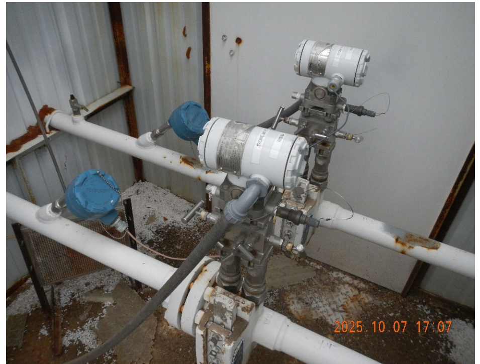
8. Gas meter inside meter shed.
