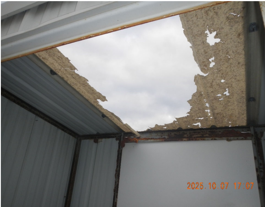
7. Damage to Meter Shed roof.
