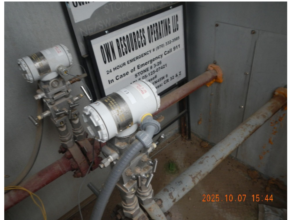
6. Gas meter inside meter shed.
