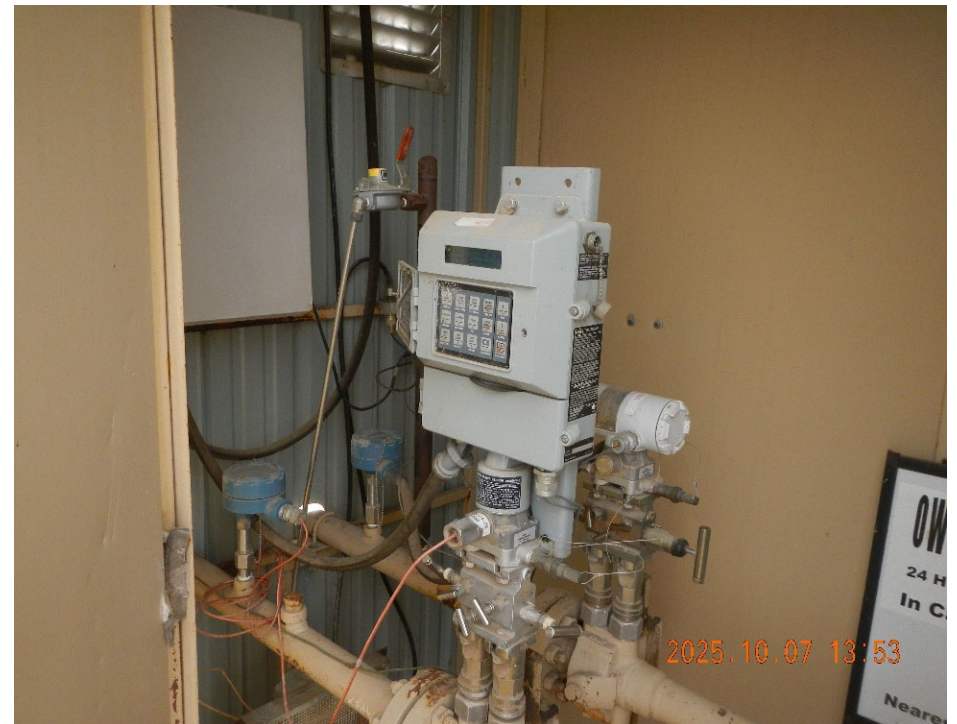
2. View of gas meter.
