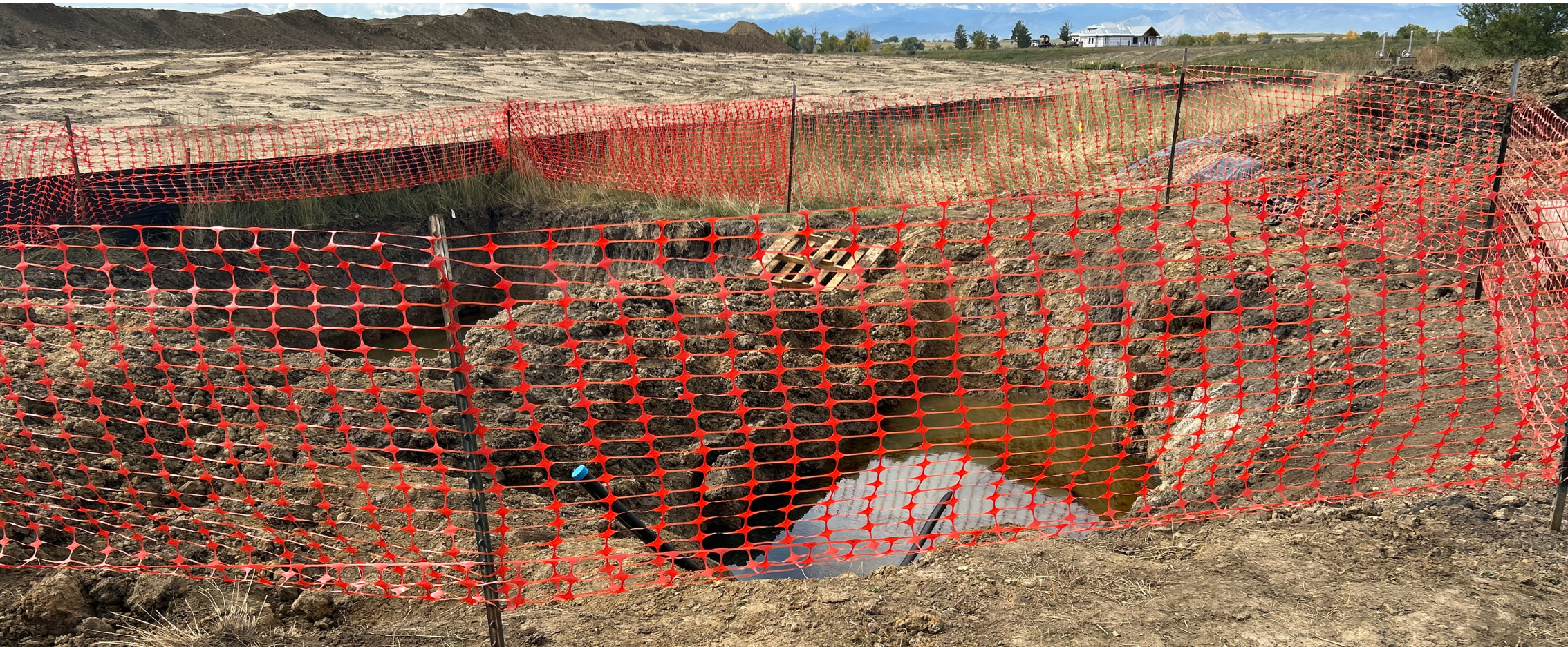
Looking at the spill location. The excavations remain open.
