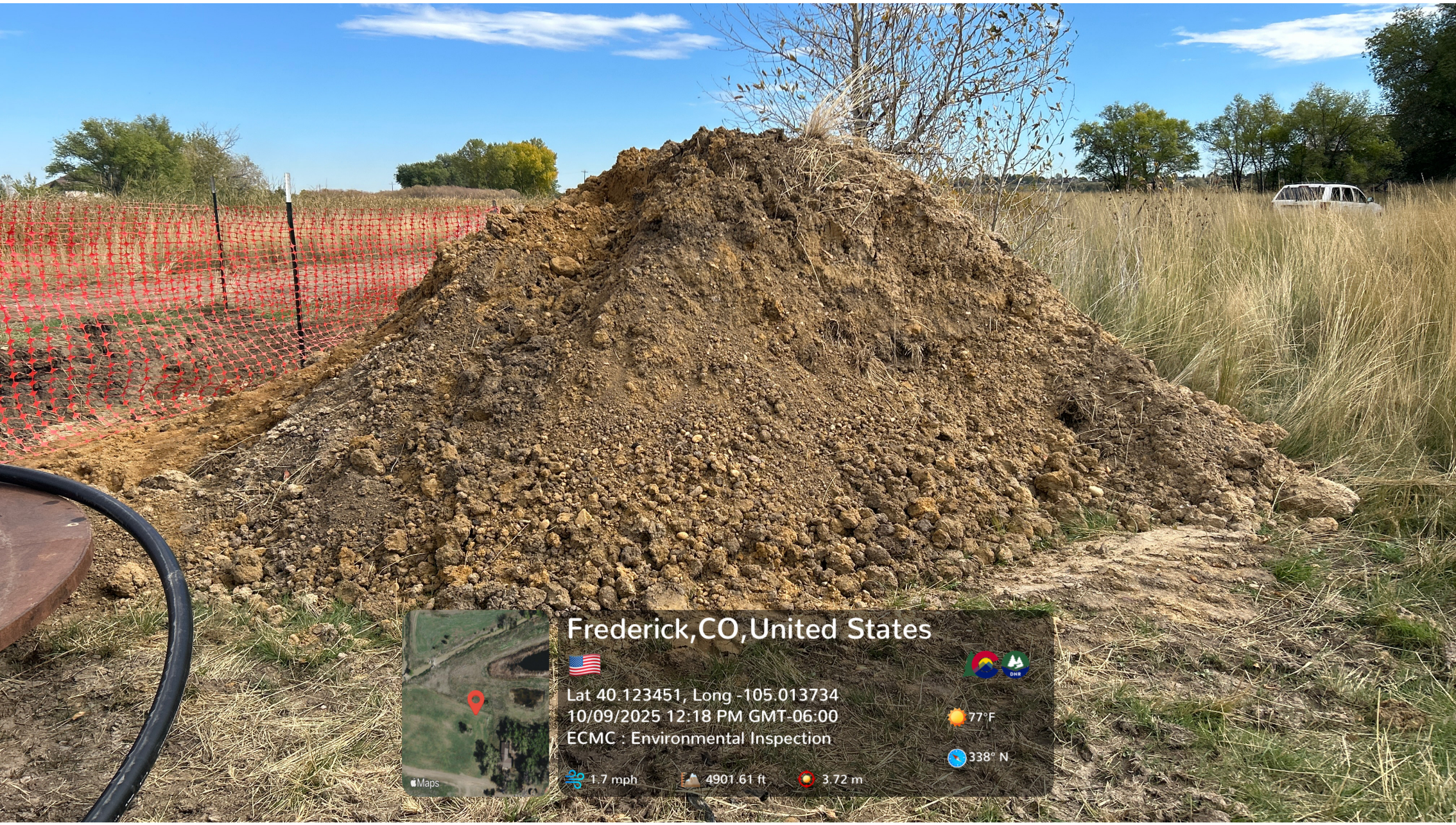
An unmarked soil stockpile with no stormwater BMPs is visible adjacent to an open excavation.
