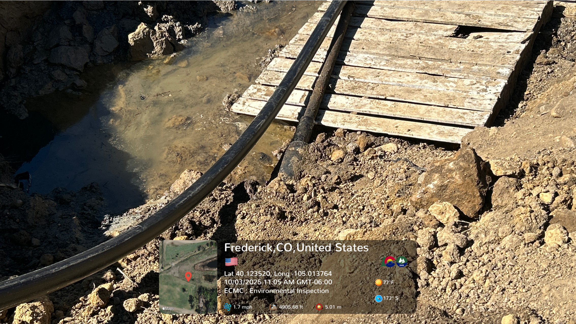
Looking at flowlines.
