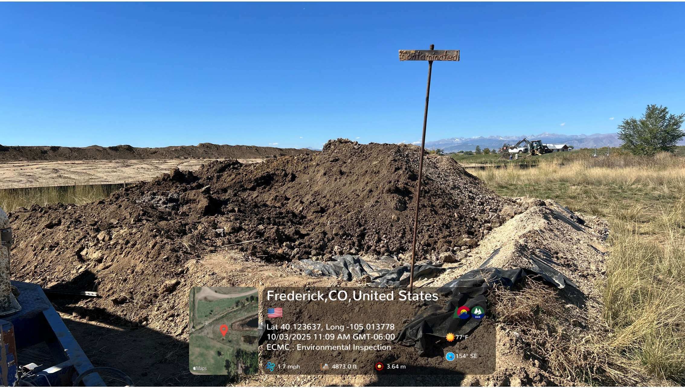
The stockpile marked "contaminated" remains on location. A liner is visible but has been compromised by holes/tears; soil has spilled outside of containment.
