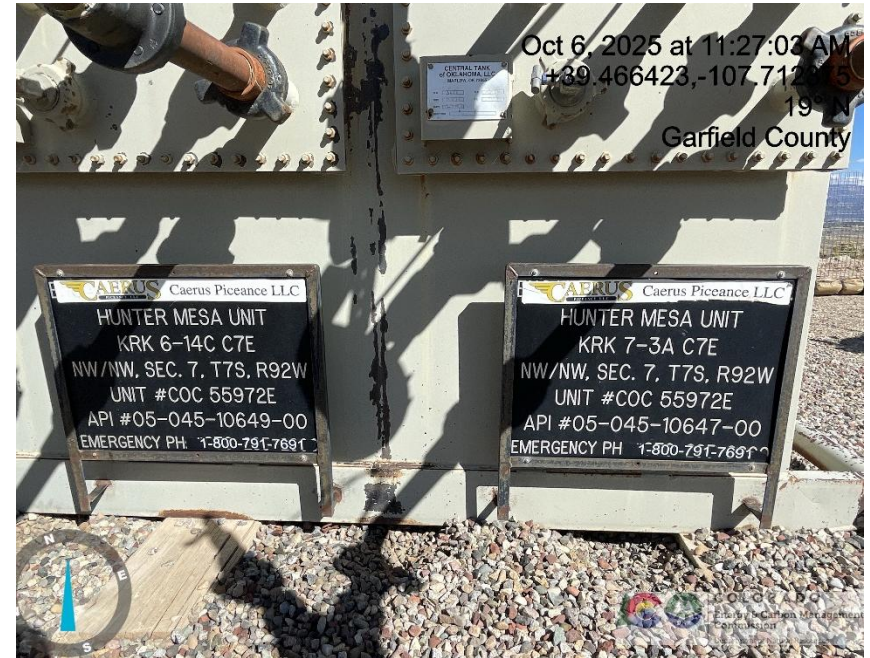
Photo # 3965 Signs at separators have previous operators name
