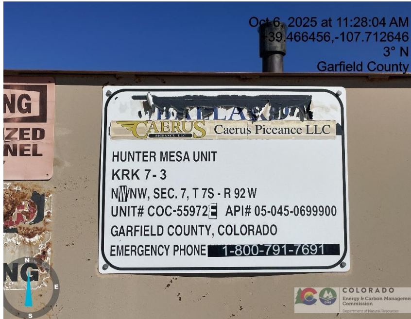
Photo # 3970 Sign at separator has previous operators name
