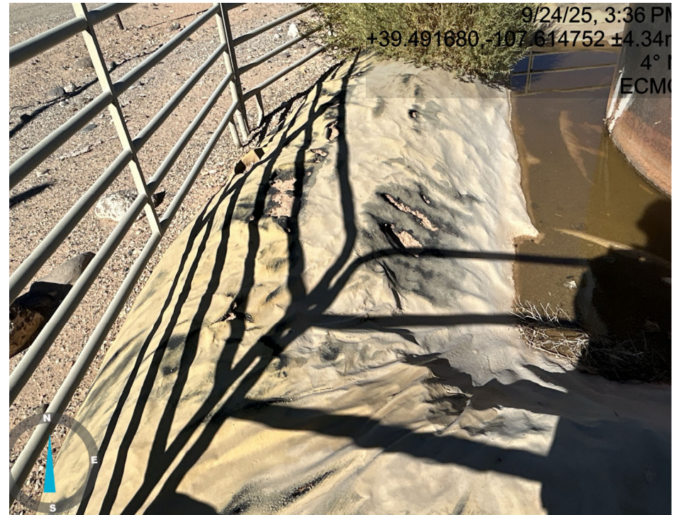
Tank liner has multiple areas with holes
