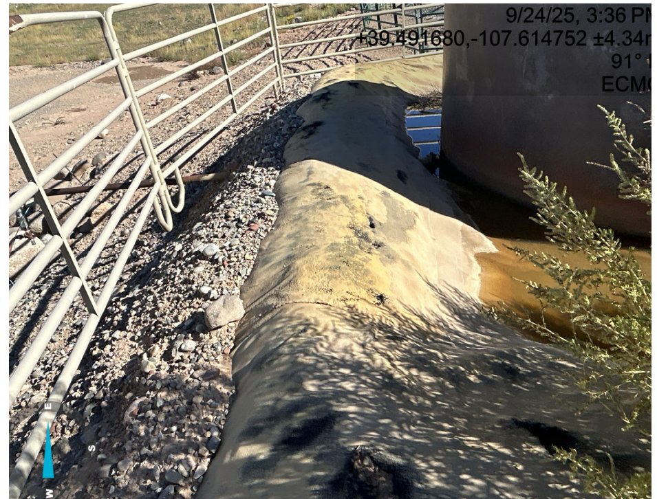
Tank liner has multiple areas with holes
