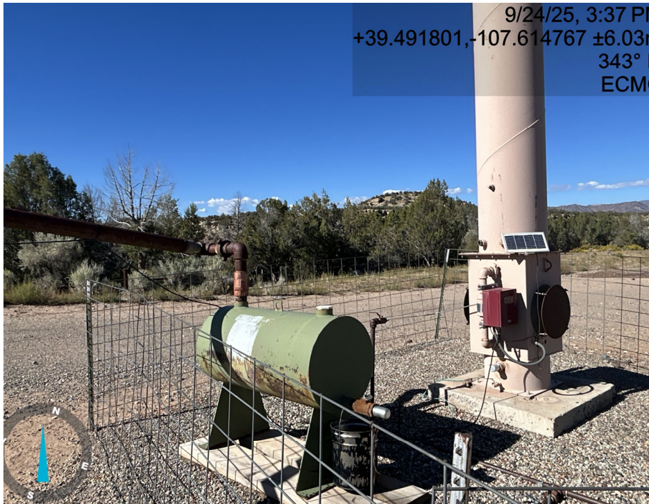
ECD is not running and not metered
