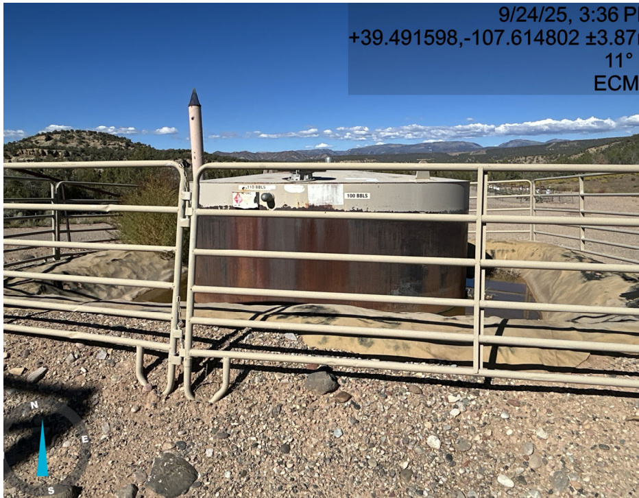
Tank liner has multiple areas with holes
