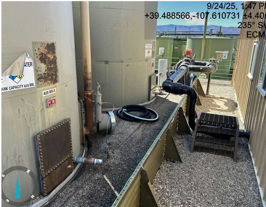
Stored hose and tank labeling falling off
