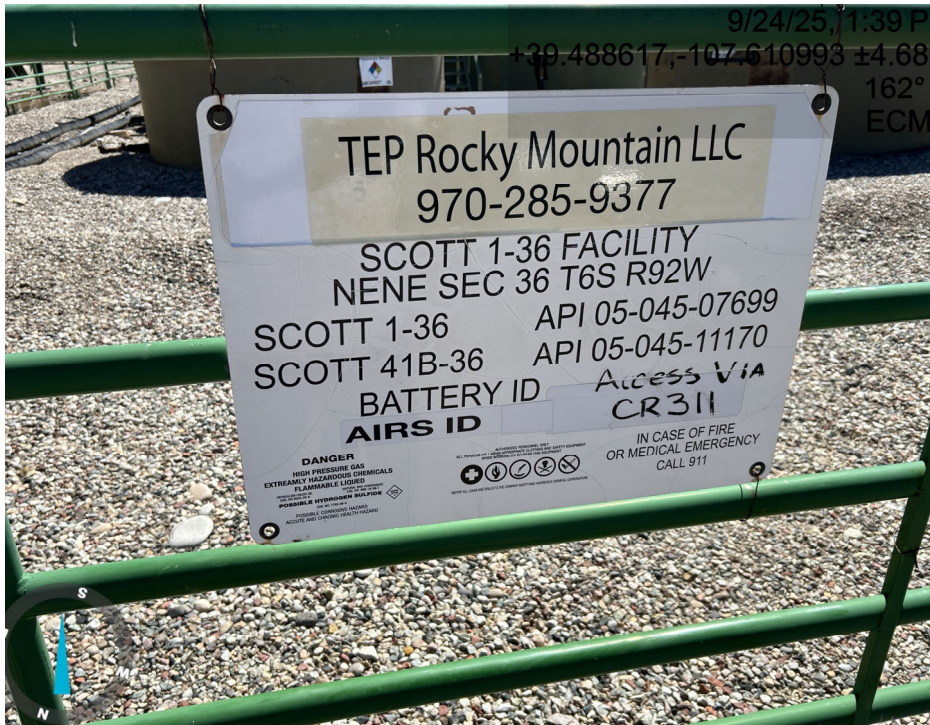
Battery sign is lacking a well
