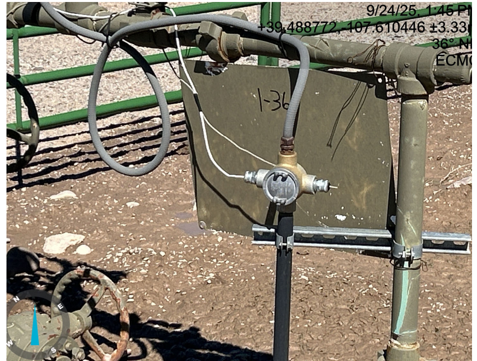
Well sign lacks information
