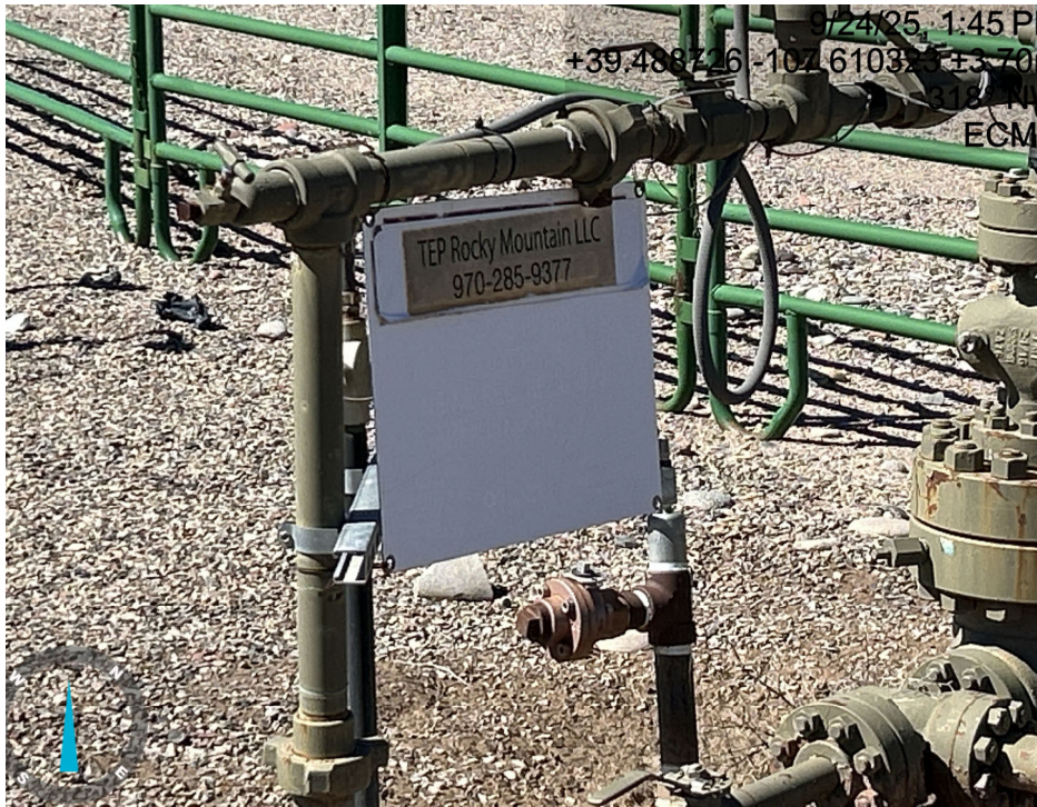
Well sign lacks information
