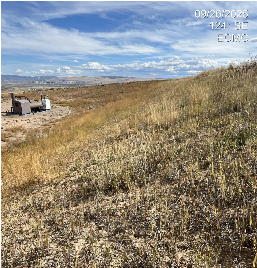
Photo 3. Photo taken mid-slope of the cut slope on the western portion, facing southeast.
