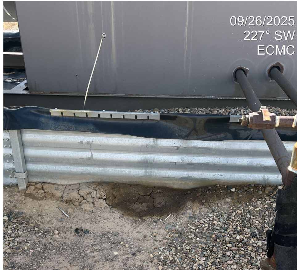
Photo 12. Photos 12-13 taken at the separator equipment along the outside eastern perimeter, illustrating stained soils.
