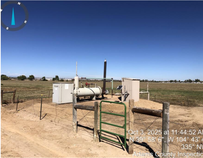
Photo #3 Separator & meter.
