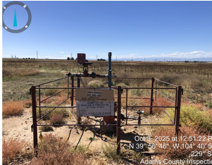
Photo #3 Well head.
