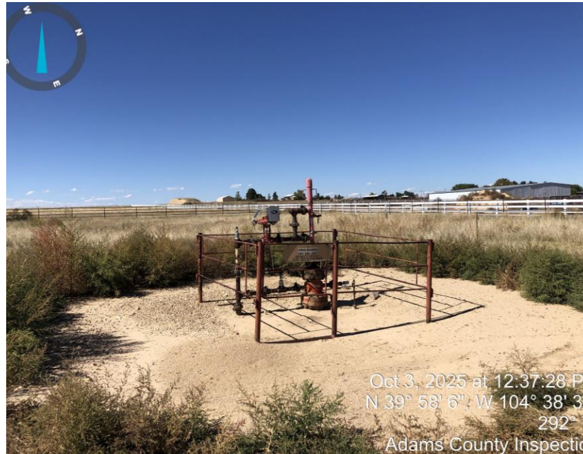
Photo #3 Well head.
