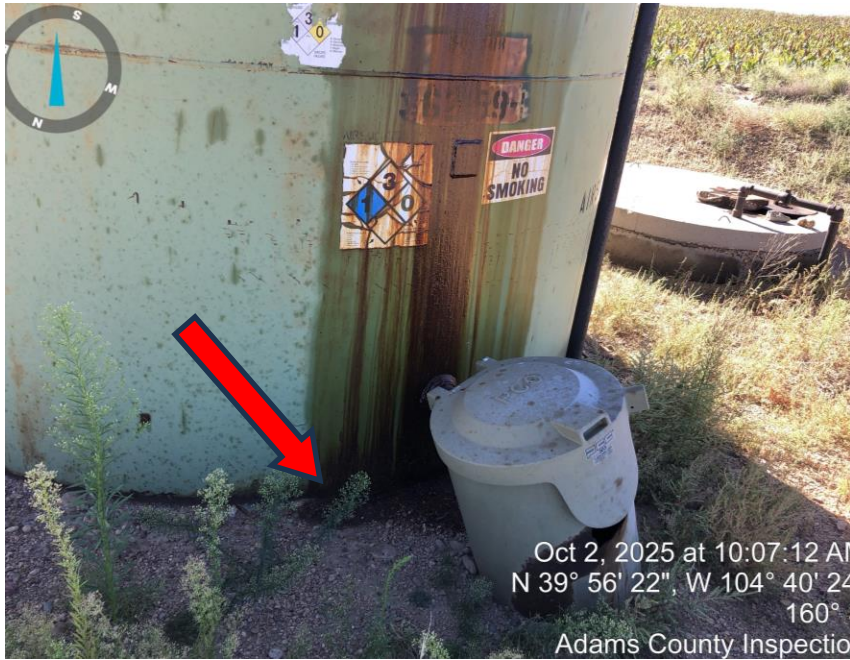
Photo #3 stained soil
