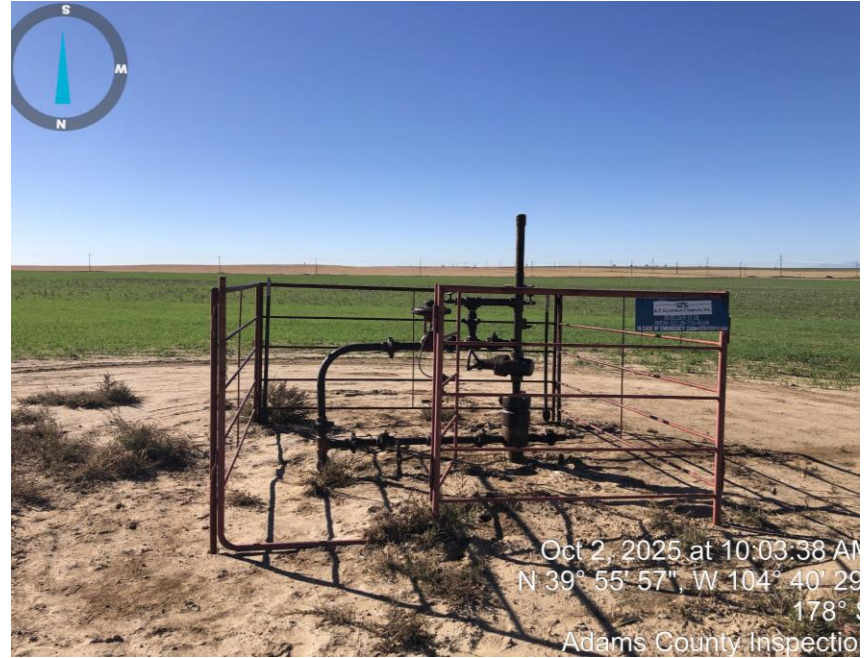
Photo #3 Well head.
