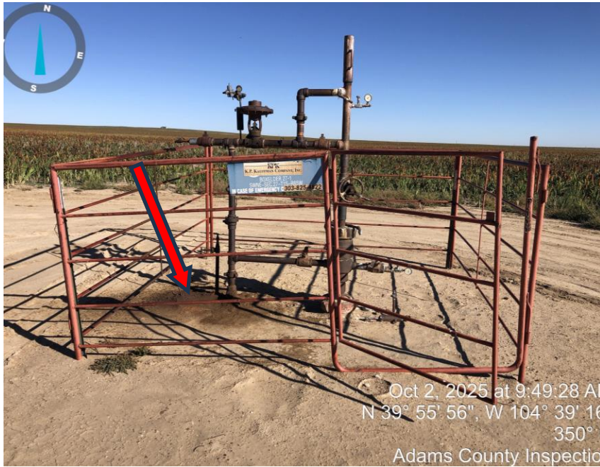
Photo #3 Well head, stained soil.
