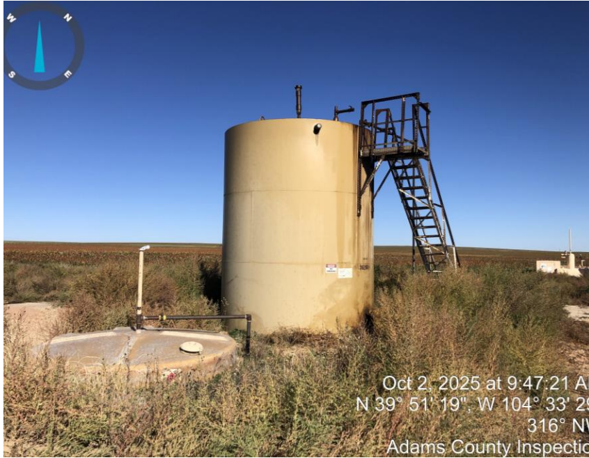
Photo #1 Tanks & weeds.
