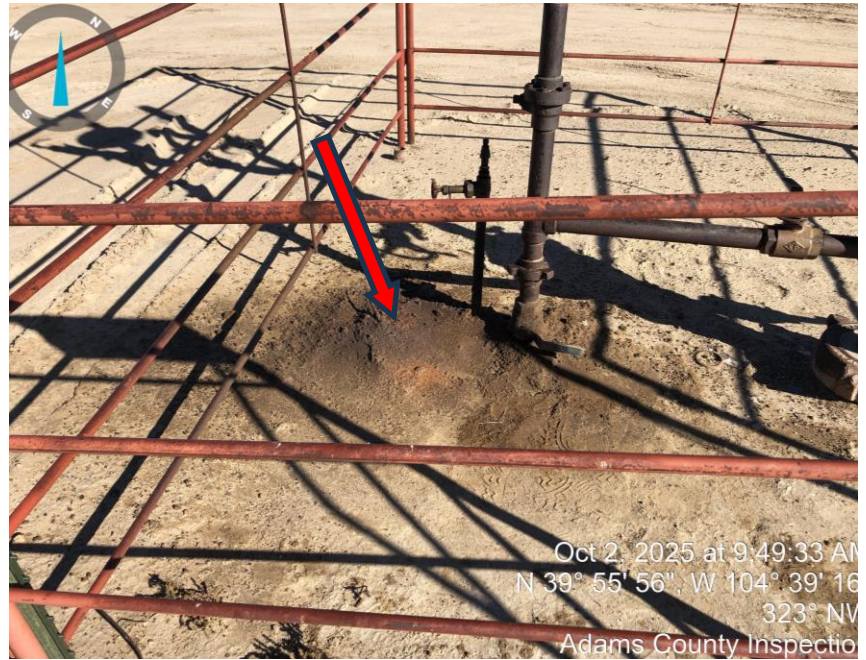
Photo #4 Well head, stained soil.
