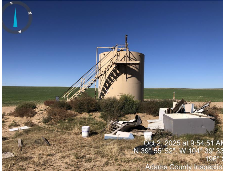
Photo #2 Tanks, weeds & trash.
