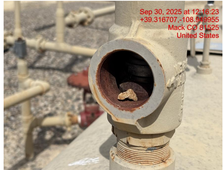
PRV Terminates in Unsafe Manner/Debris in Vent – Photo #00941
