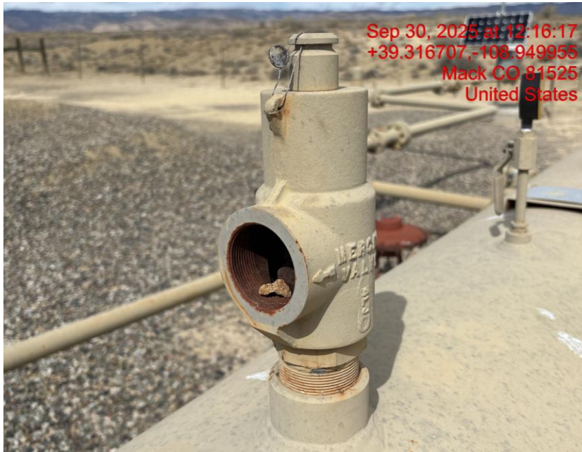
PRV Terminates in Unsafe Manner – Photo #00940
