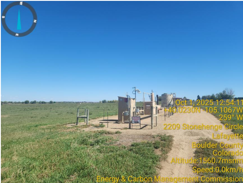
Photo 1 Tank battery location.
