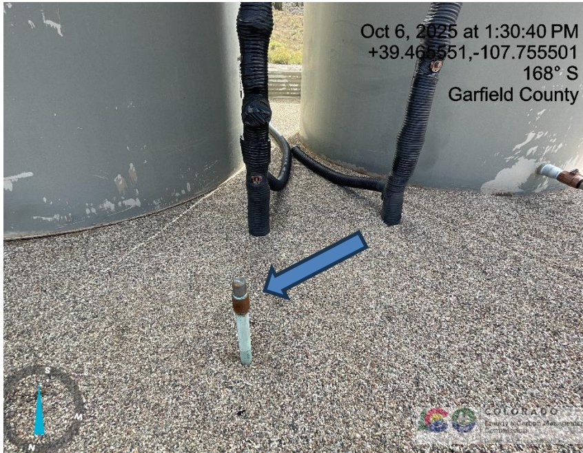
Photo # 4246 Unused flowline lacks lockout tagout (OOSLAT)
