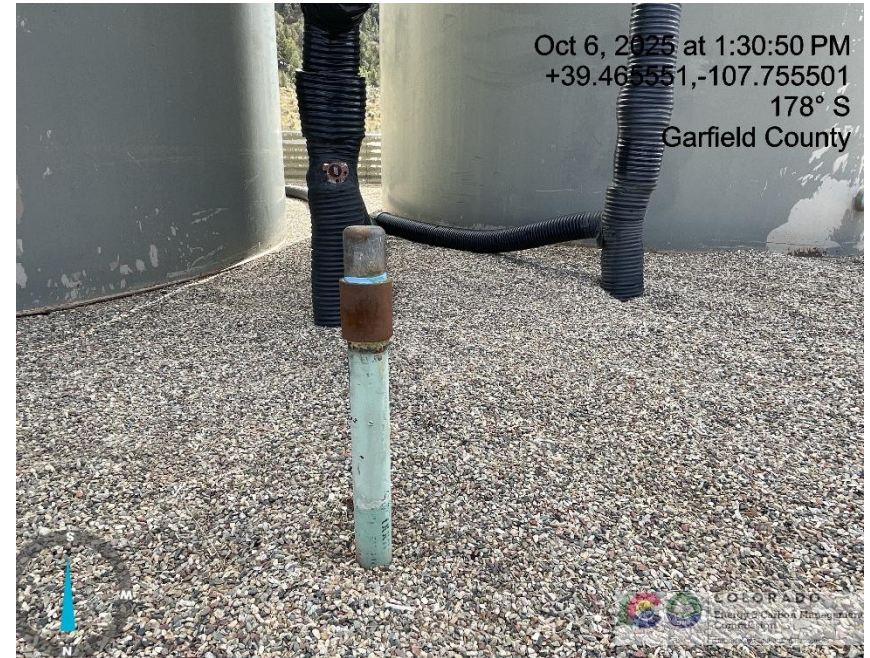
Photo # 4247 Unused flowline lacks lockout tagout (OOSLAT)
