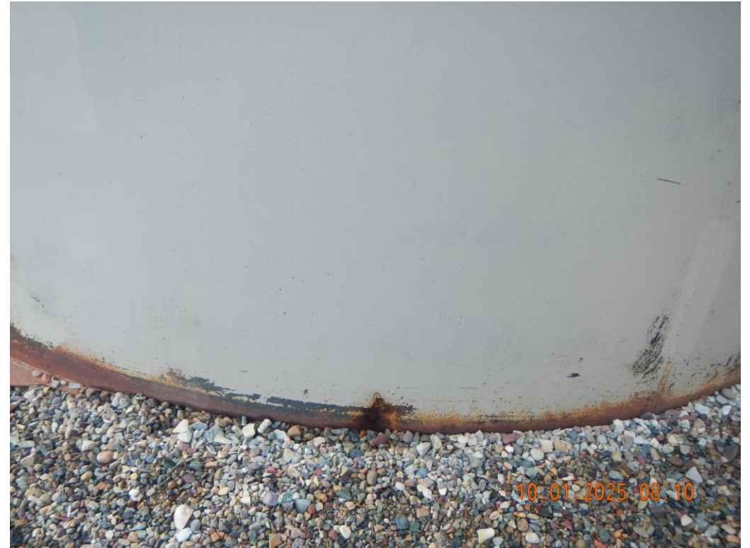
Seep at the bottom tank.
