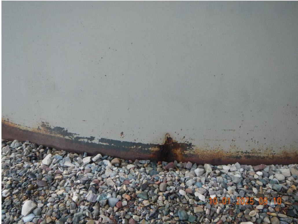
Seep at the bottom tank.
