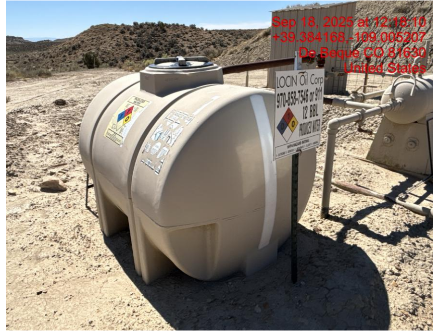
No Secondary Containment Around Tank – Photo #00857
