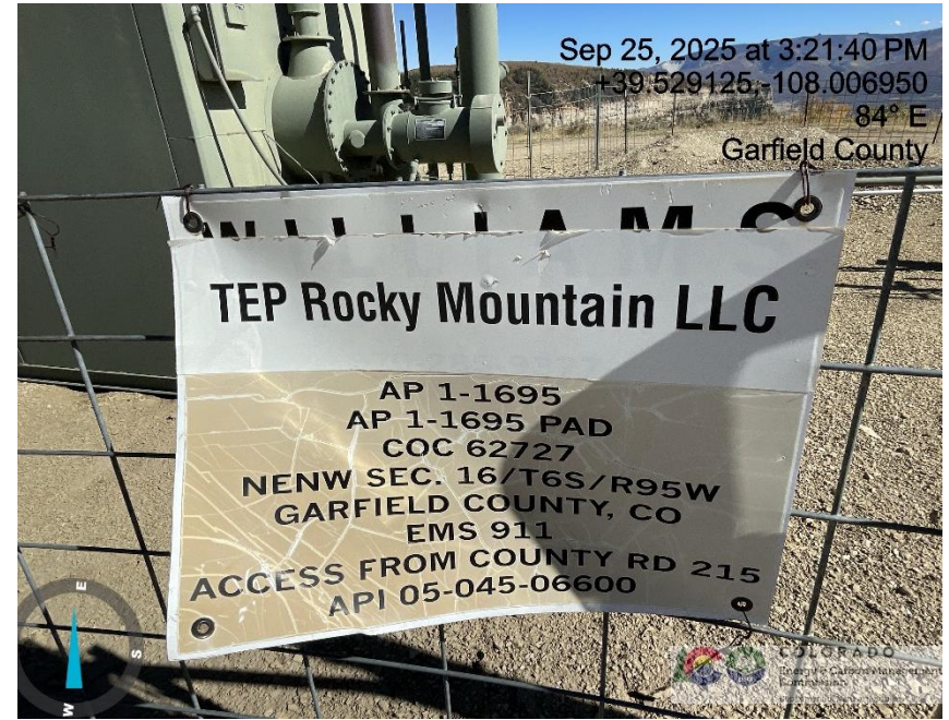
Photo # 3208 Operator # not visible on wellhead sign
