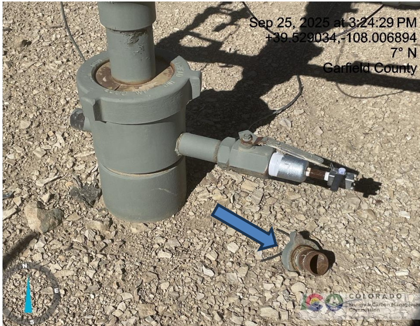
Photo # 3209 Open ended pipe near wellhead/wildlife hazard /available for entry by wildlife
