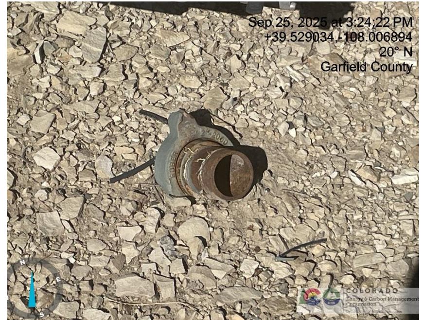
Photo # 3210 Open ended pipe near wellhead/wildlife hazard /available for entry by wildlife
