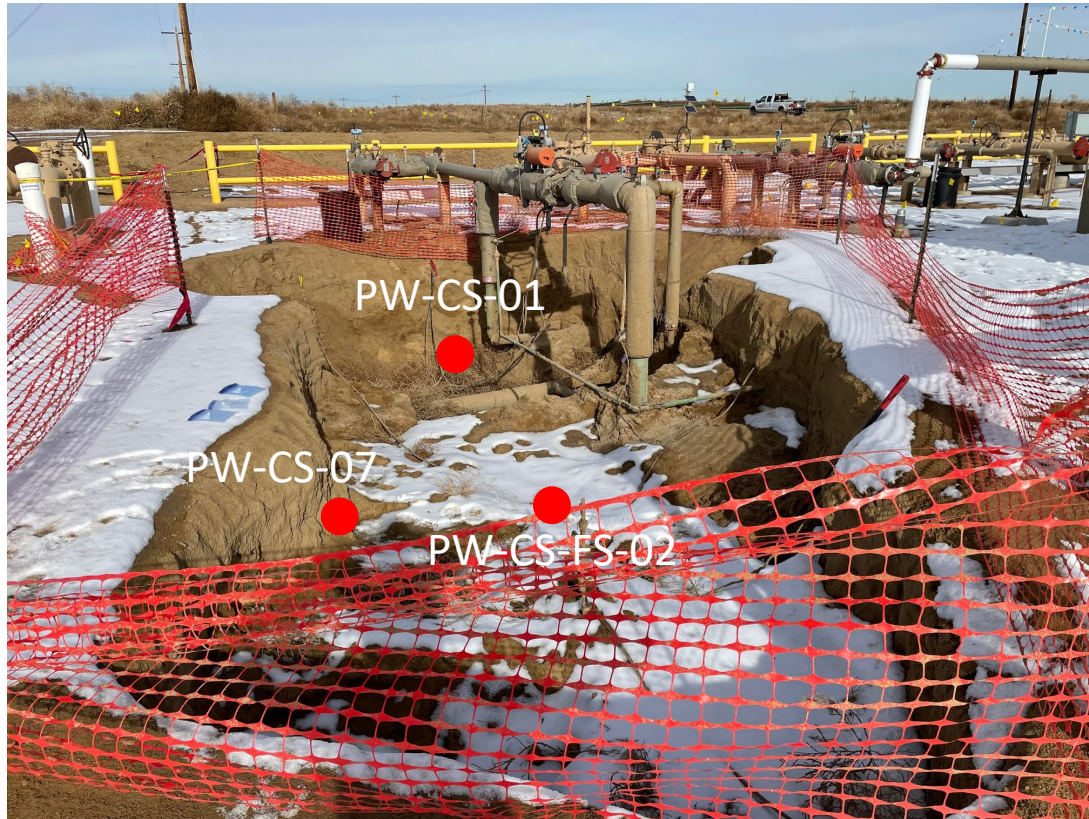
Looking north No petroleum hydrocarbon staining or odor observed Samples collected: PW-CS-01@8' – 1.7 ppm-v PW-CS-07@3' – 7.5 ppm-v PW-CS-FS-02@4' – 4.3 ppm-v
