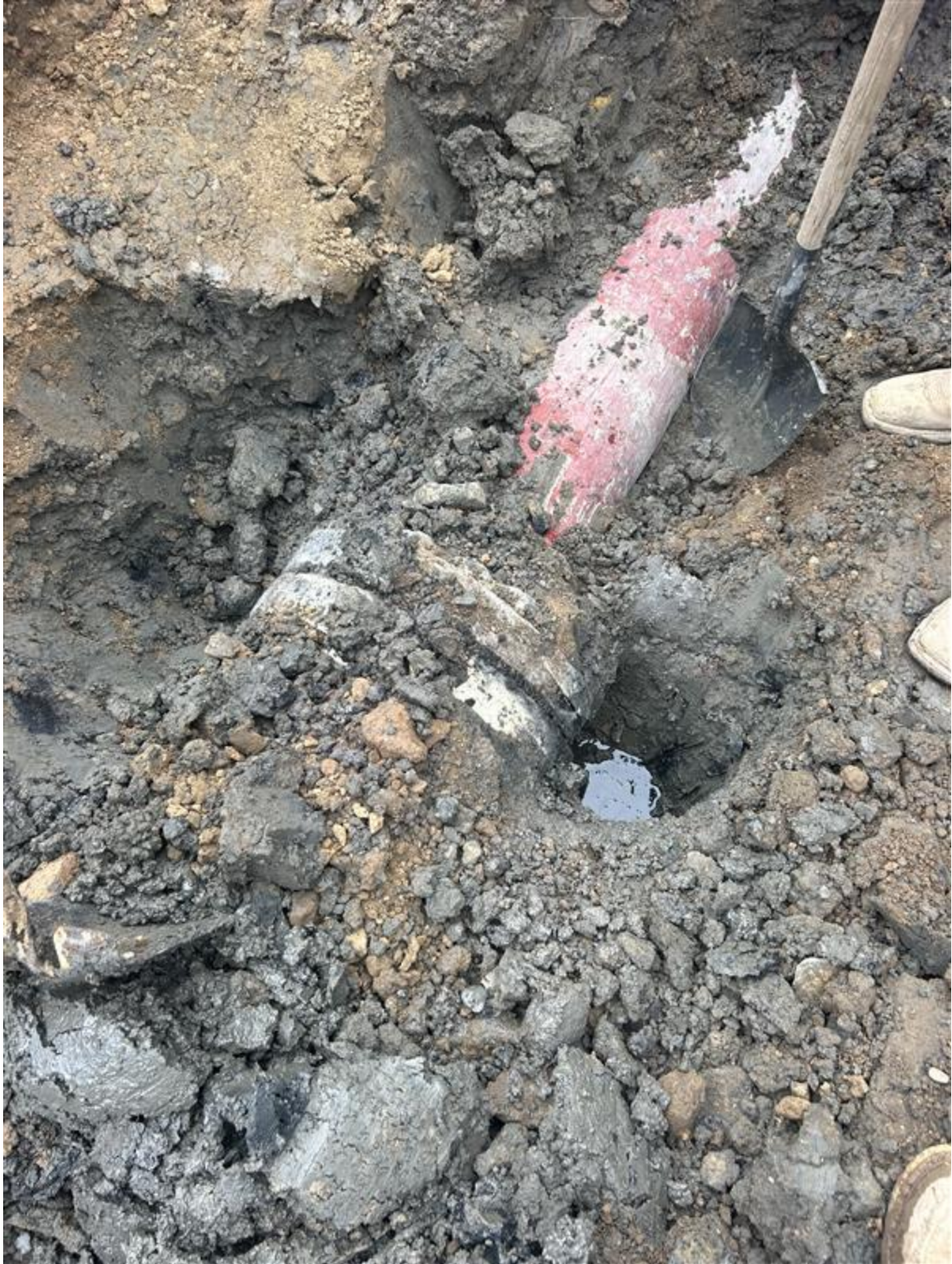
Buried leaking pipeline flange.
