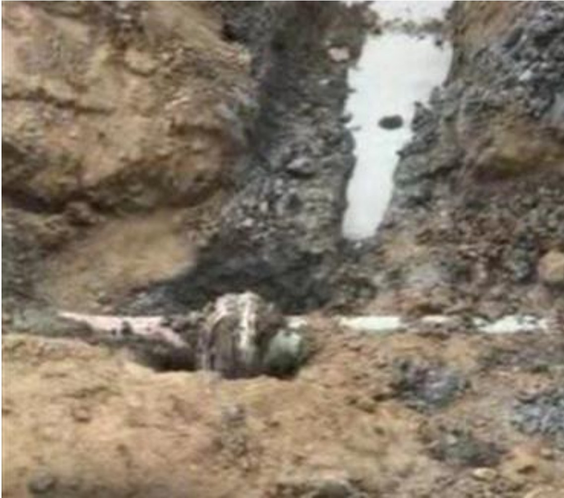
Groundwater migrating into pipeline excavation.
