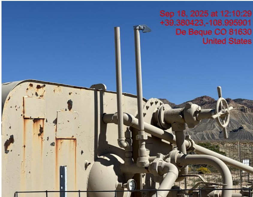
Uncovered PRV Vent – Photo #00849
