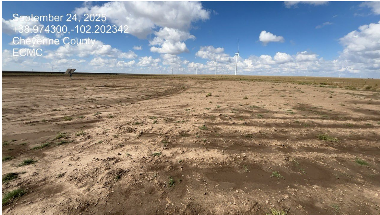
Photo 6. North side of the location facing west. The location has been recontoured but it does not appear reseeding has been performed.
