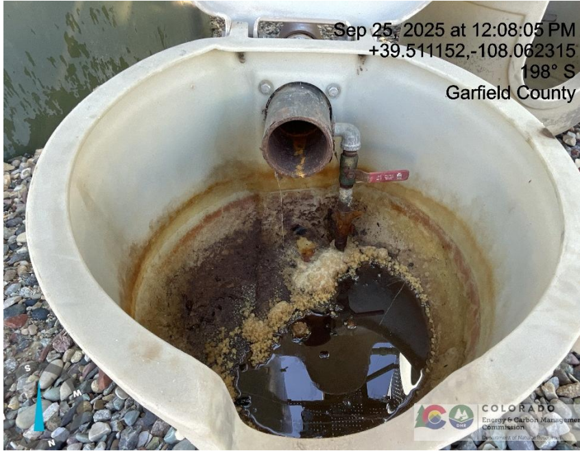
Photo # 2542 Open ended load line
