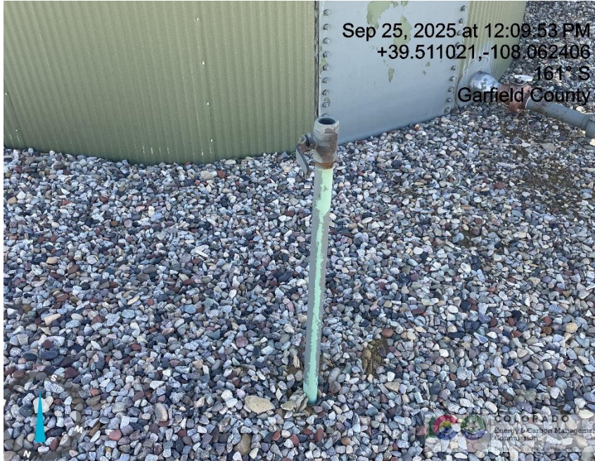
Photo # 2524 Unused flowline lacks lockout tagout (OOSLAT)
