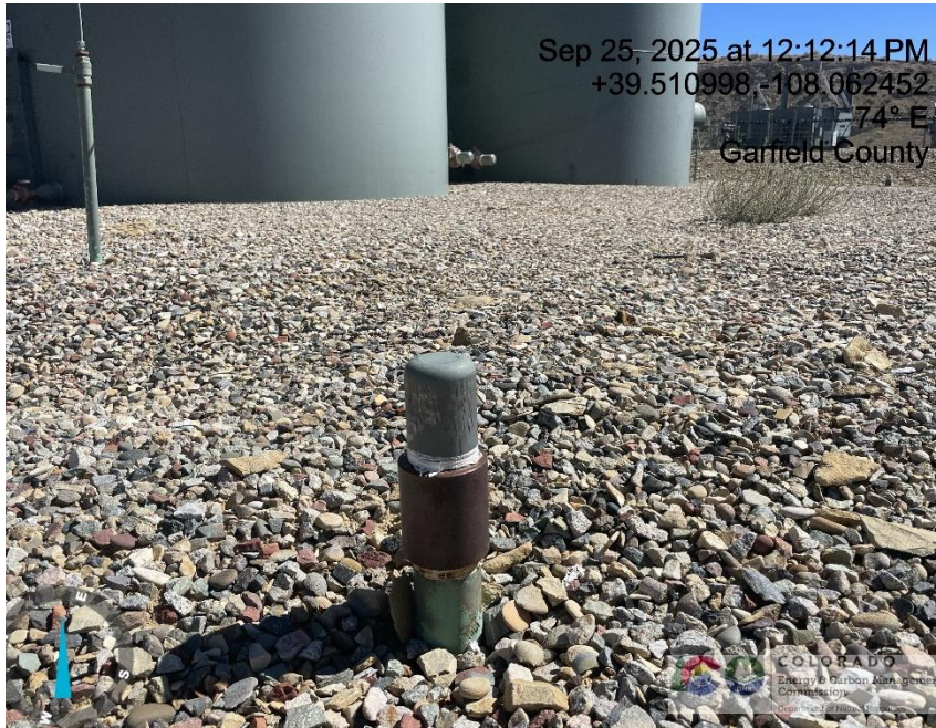
Photo # 2532 Unused flowline lacks lockout tagout (OOSLAT)
