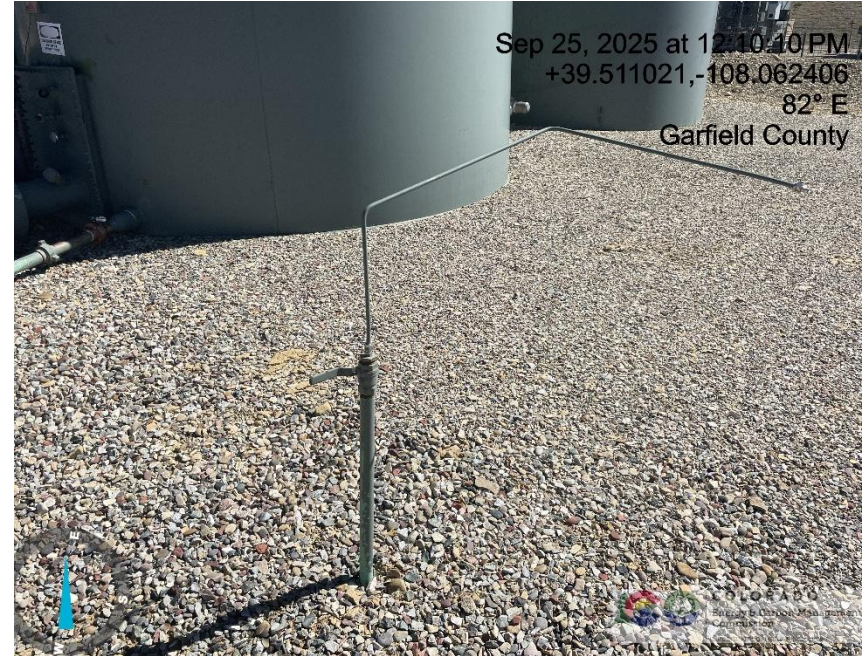
Photo # 2525 Unused flowline lacks lockout tagout (OOSLAT)
