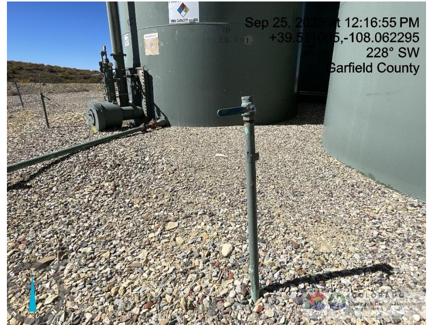
Photo # 2533 Unused flowline lacks lockout tagout (OOSLAT)
