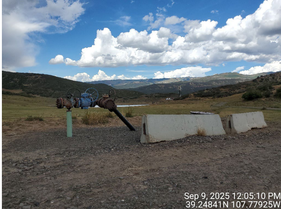
Riser with valves (blinded)
