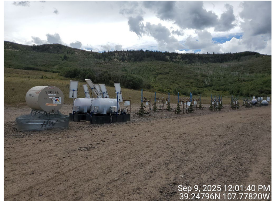
Wellheads with signs and Chemical Injectors
