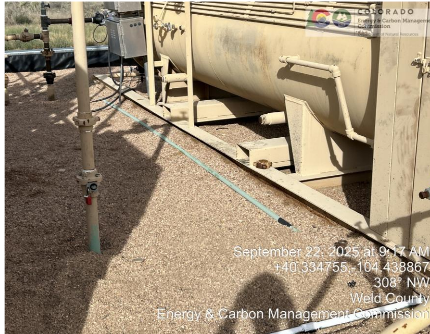
Unused Equipment “tubing”
