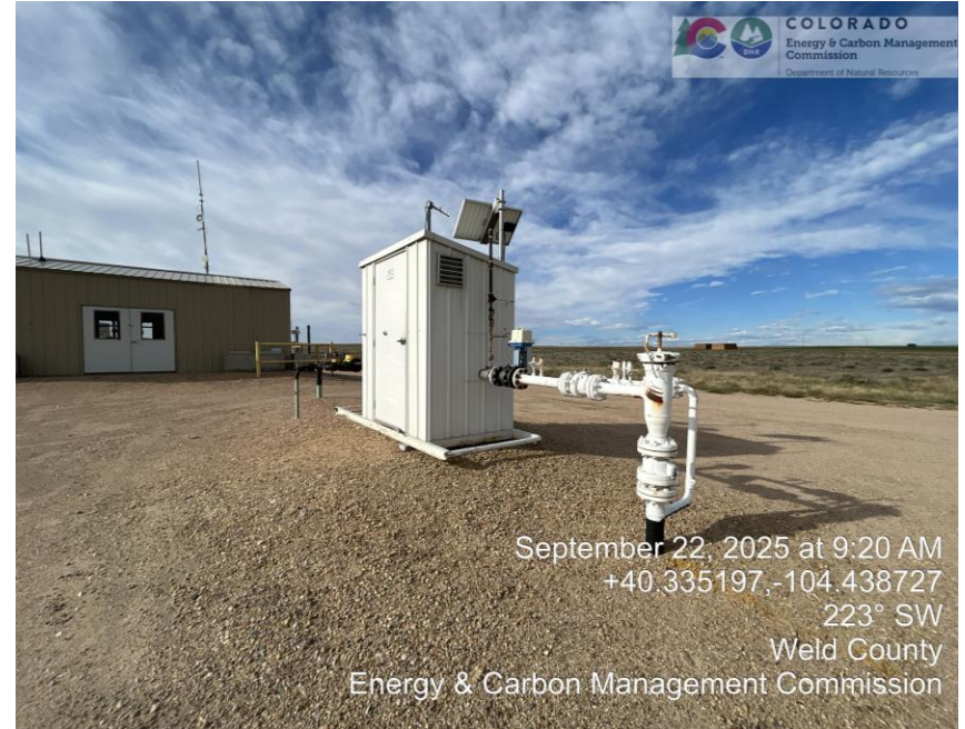
Gas Meter Run
