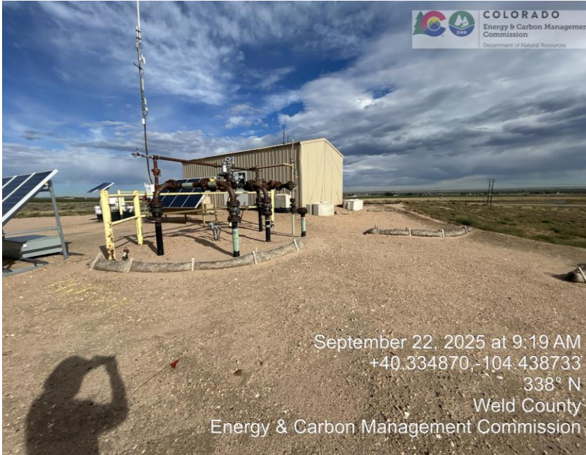
Waddles and Gaslift skid
