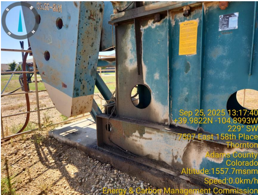
Photo 11 Leaking gasket on the pumpjack.
