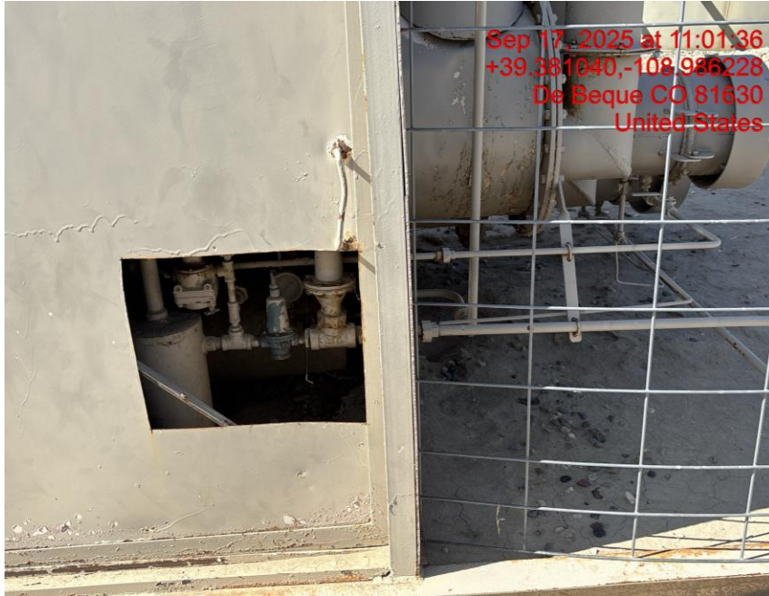
Wildlife Entry Hazard – Photo #00812
