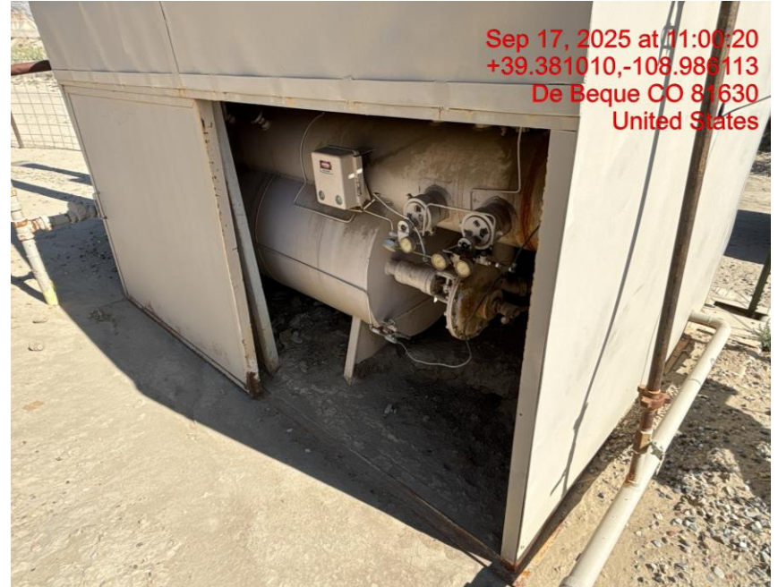
Wildlife Entry Hazard – Photo #00809
