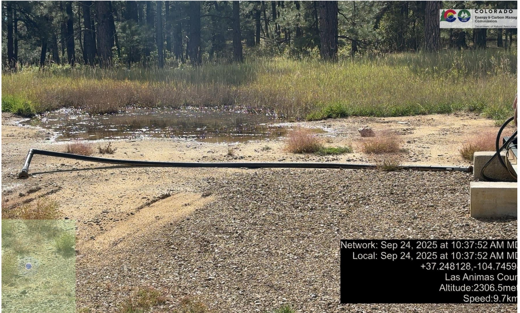
PHOTO 5: THE STORMWATER POOLING ON LOCATION SHOULD BE DRAINED. INSTALL AND MAINTAIN BMP'S TO PREVENT STORMWATER POOLING ON LOCATIONS PER 1002 SERIES RULES. CA DATE 10-24-2025.
