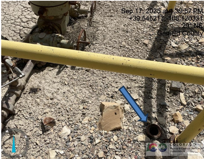
Photo # 710 Open ended piping near wellhead/wildlife hazard/available for entry by wildlife
