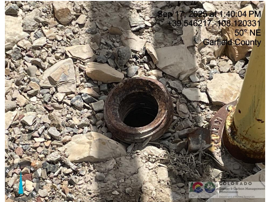
Photo # 711 Open ended piping near wellhead/wildlife hazard/available for entry by wildlife
