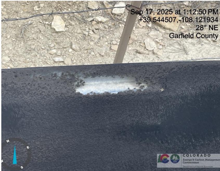
Photo # 600 Hole in secondary containment liner/liner needs maintenance
