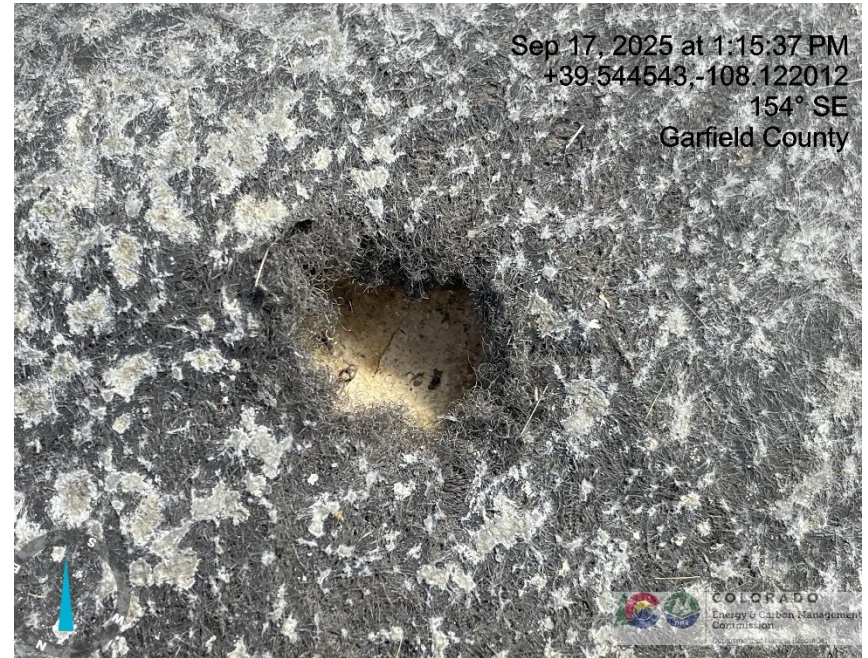
Photo # 609 Hole in secondary containment liner/liner needs maintenance
