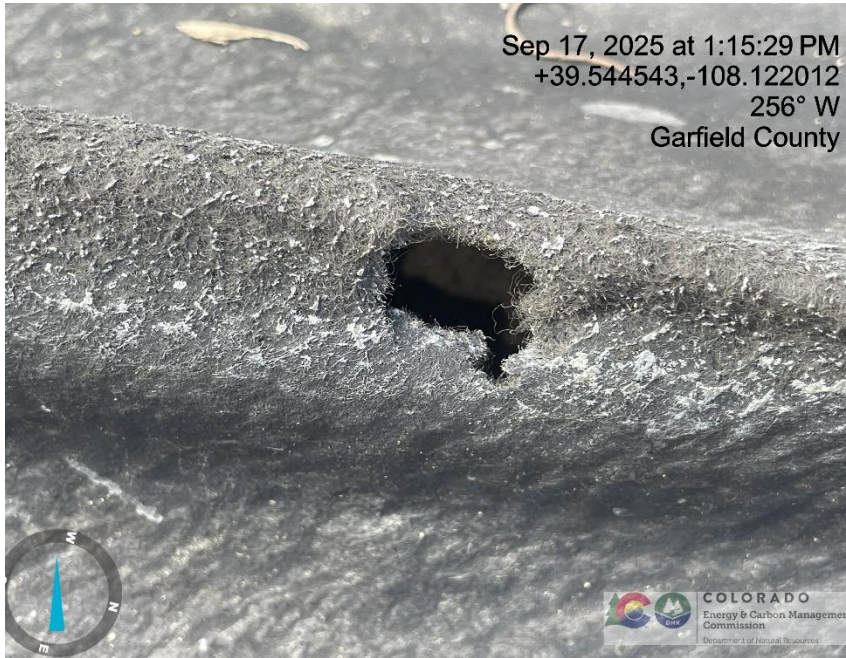
Photo # 608 Hole in secondary containment liner/liner needs maintenance
