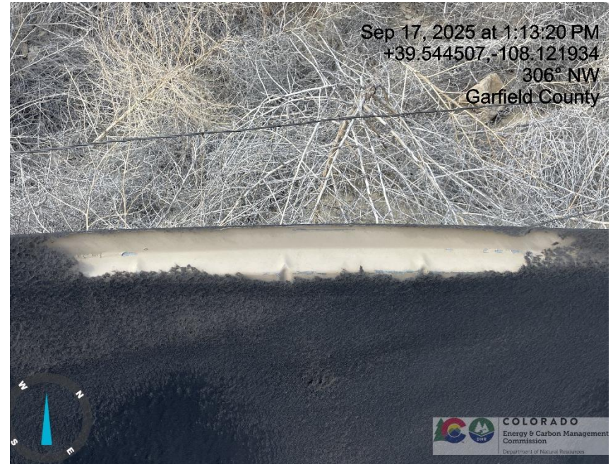
Photo # 603 Hole in secondary containment liner/liner needs maintenance
