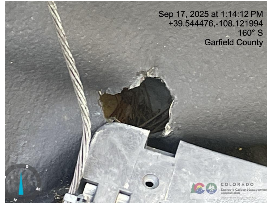
Photo # 605 Hole in secondary containment liner/liner needs maintenance
