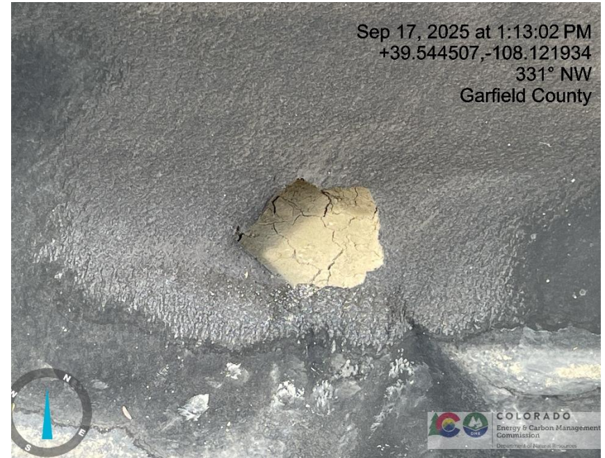
Photo # 601 Hole in secondary containment liner/liner needs maintenance
