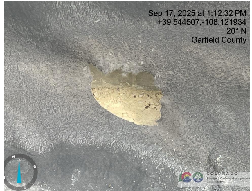
Photo # 597 Hole in secondary containment liner/liner needs maintenance
