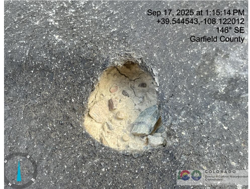
Photo # 607 Hole in secondary containment liner/liner needs maintenance
