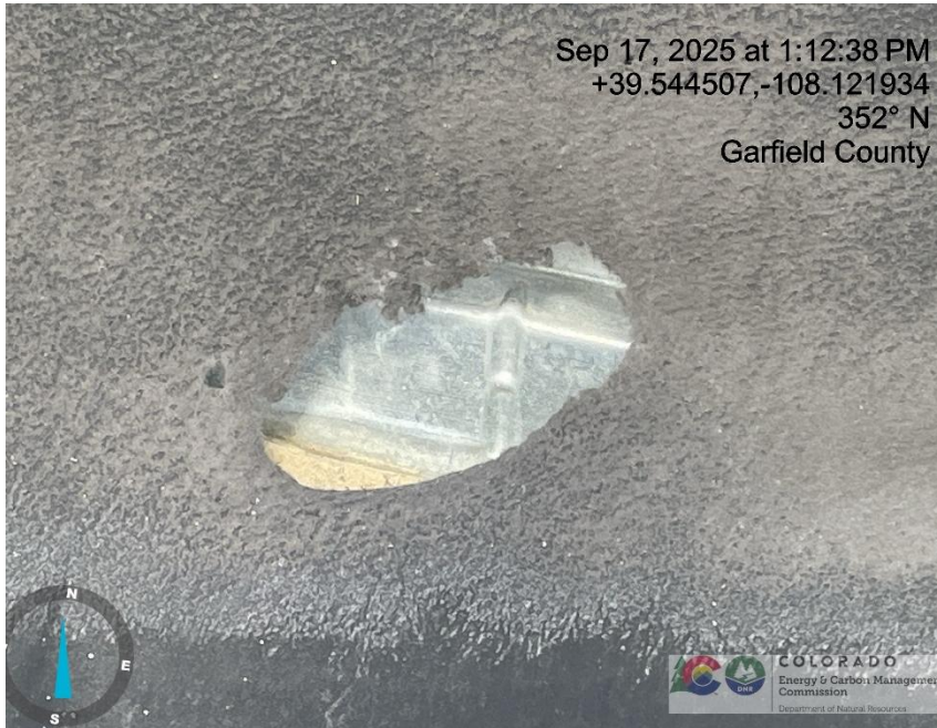
Photo # 598 Hole in secondary containment liner/liner needs maintenance
