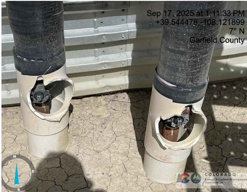
Photo # 596 Flowline heating insulation open ended/wildlife hazard/available for entry by wildlife
