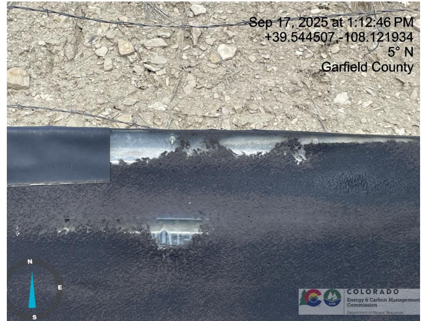
Photo # 599 Holes in secondary containment liner/liner needs maintenance
