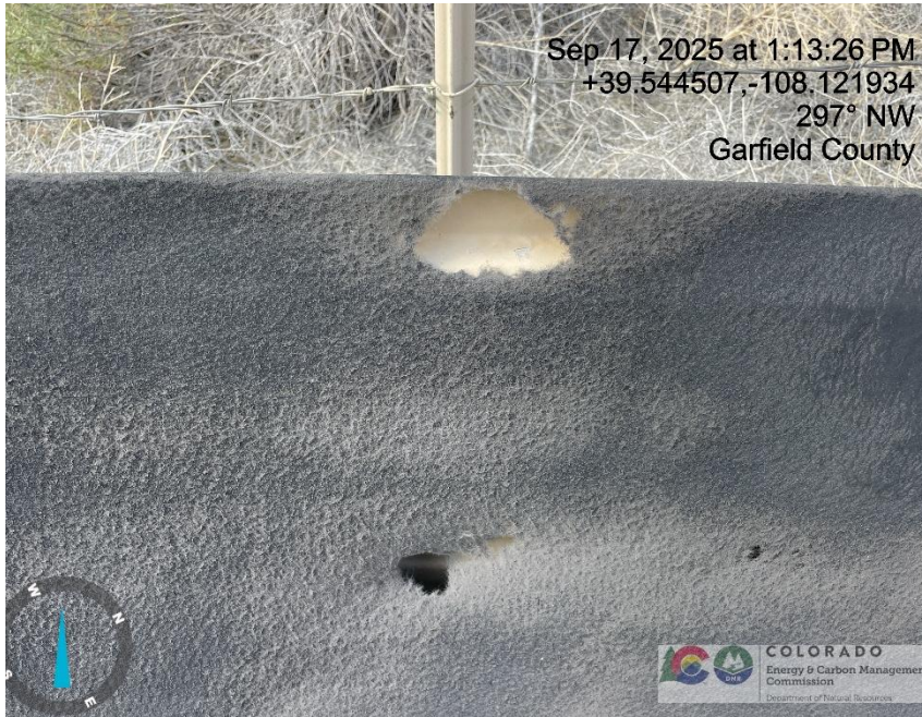
Photo # 604 Holes in secondary containment liner/liner needs maintenance
