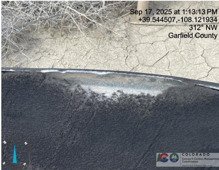
Photo # 602 Hole in secondary containment liner/liner needs maintenance
