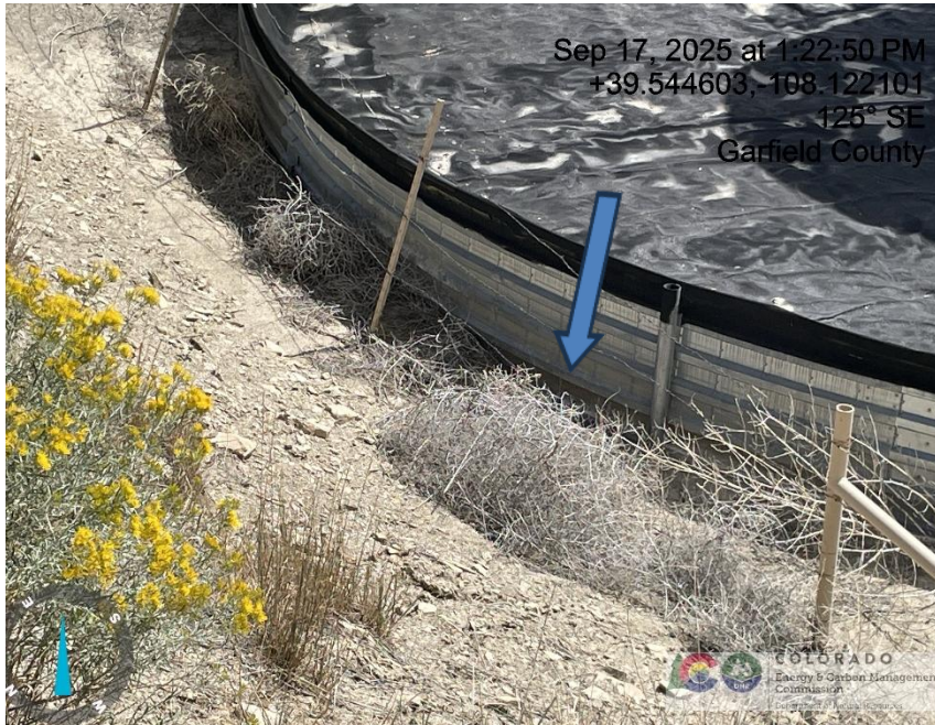
Photo # 610 Dead weeds/debris
