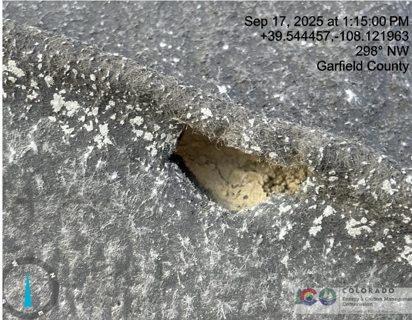
Photo # 606 Hole in secondary containment liner/liner needs maintenance
