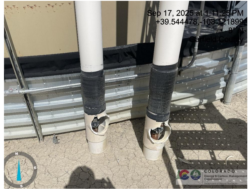
Photo # 595 Flowline heating insulation open ended/wildlife hazard/available for entry by wildlife
