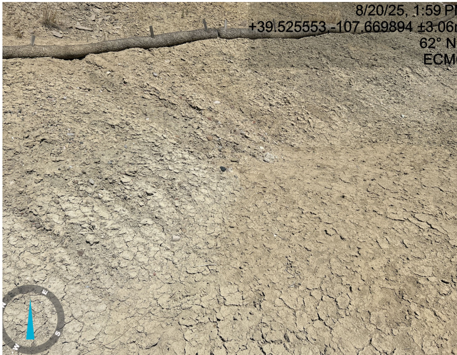
Erosion on cut slope and BMP's failing
