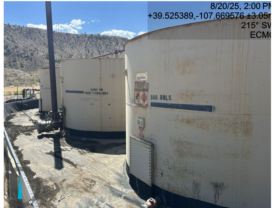
Tank signage weathered
