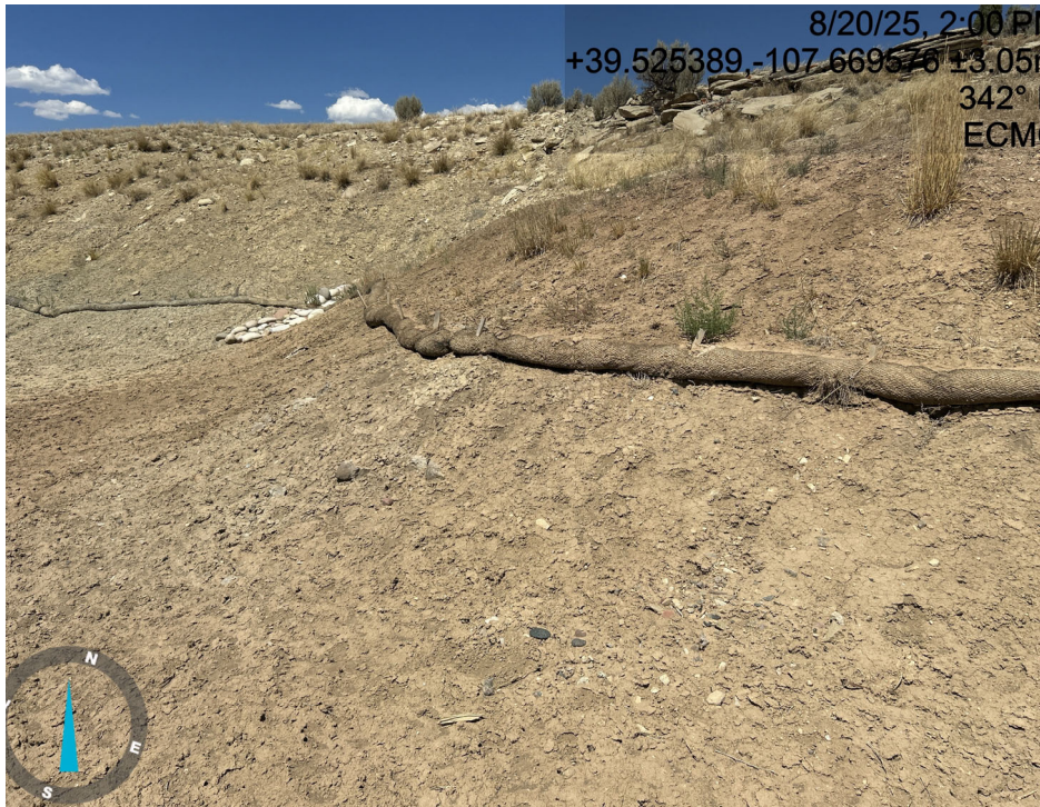
Erosion on cut slope and BMP's failing
