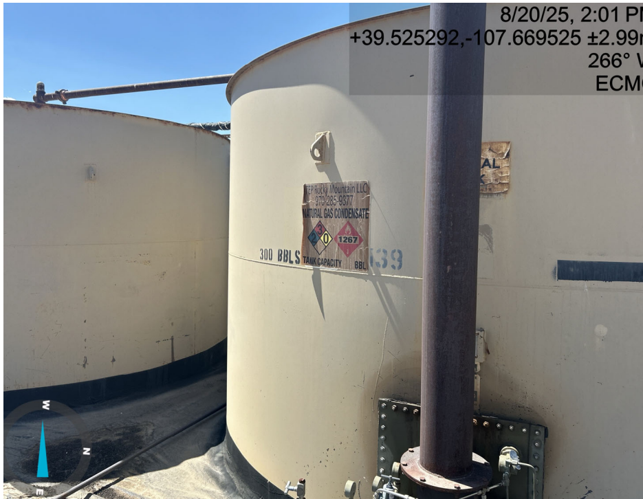
Tank signage weathered
