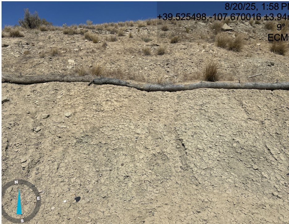
Erosion on cut slope and BMP's failing
