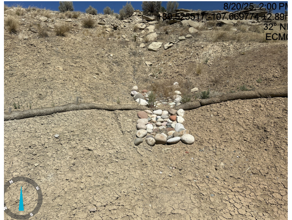
Erosion on cut slope and BMP's failing
