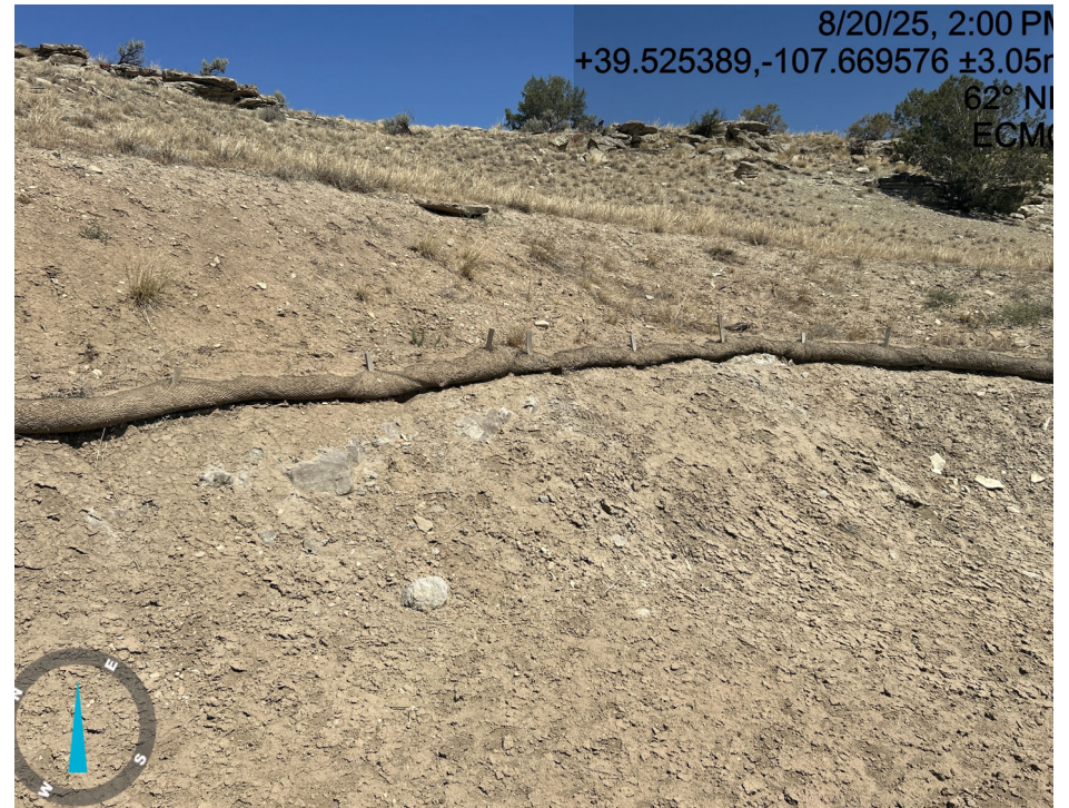
Erosion on cut slope and BMP's failing
