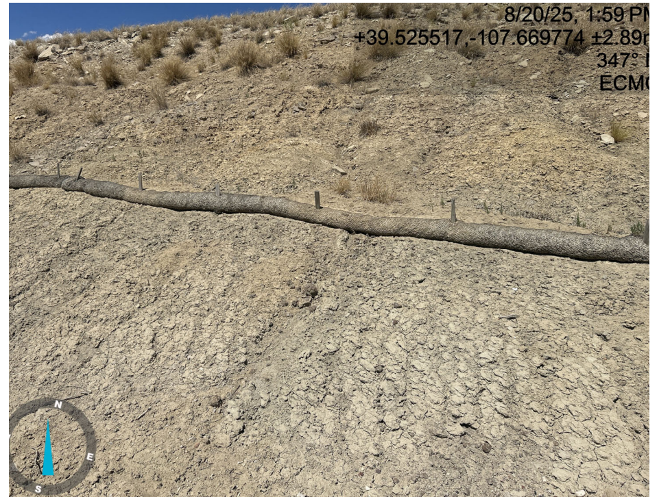
Erosion on cut slope and BMP's failing
