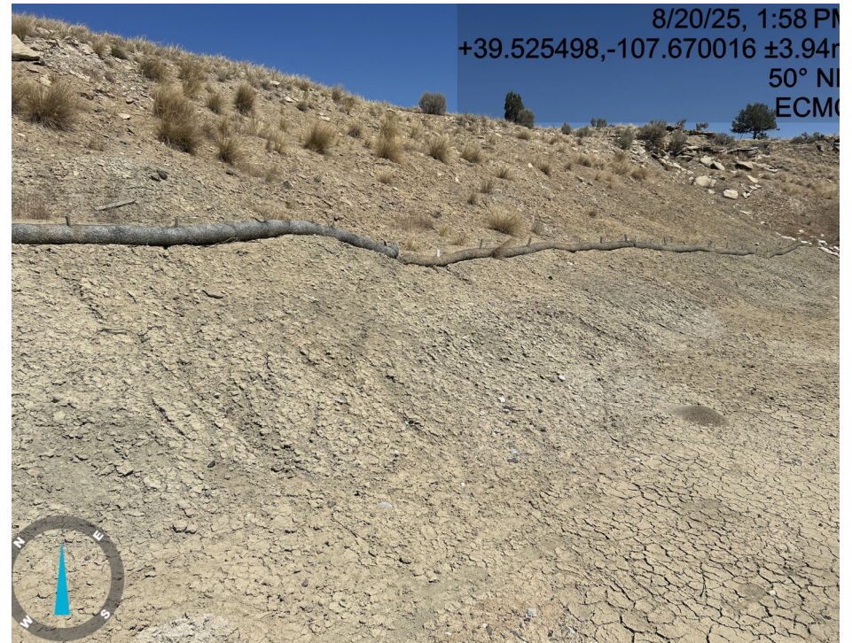
Erosion on cut slope and BMP's failing
