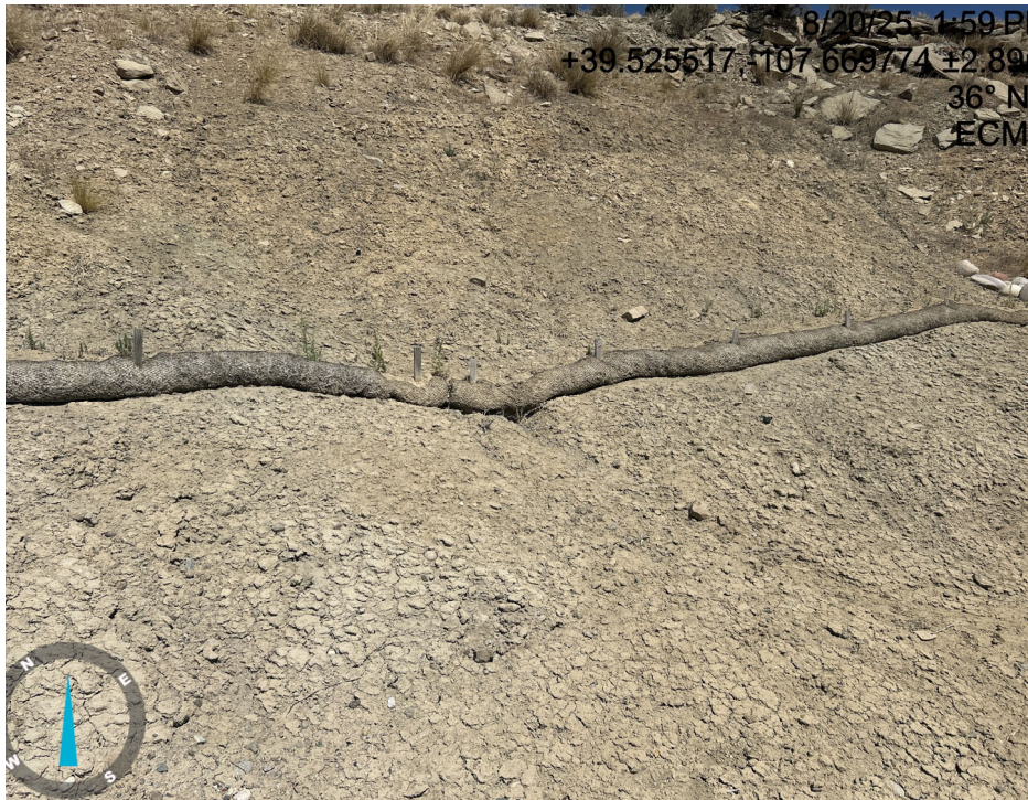
Erosion on cut slope and BMP's failing
