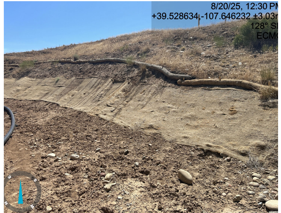
Cut slope erosion
