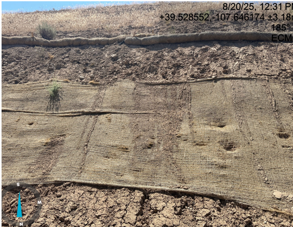
Cut slope erosion
