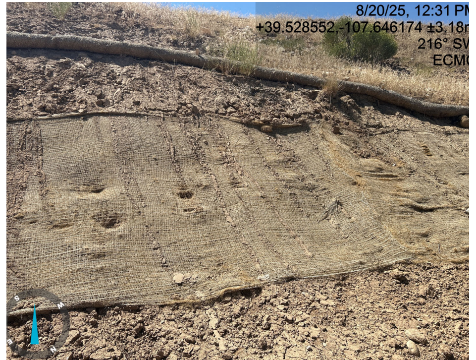
Cut slope erosion
