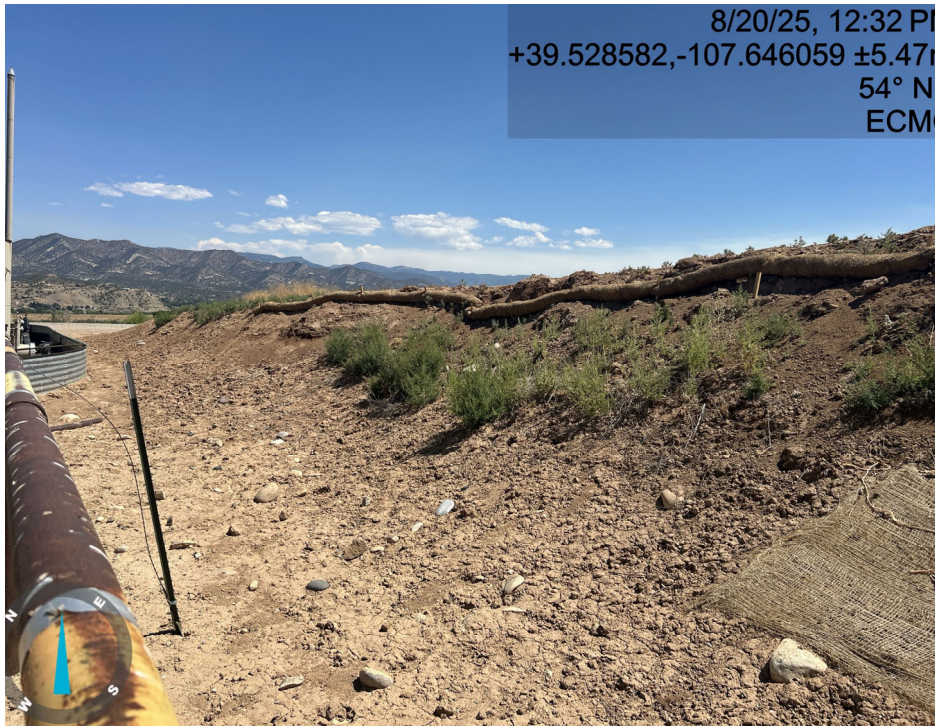
Cut slope erosion
