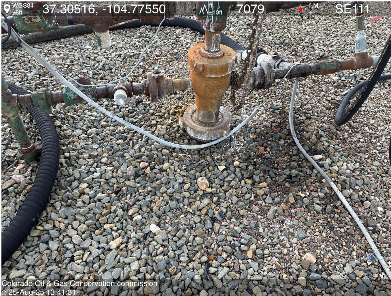
PHOTO 8: Bradenhead inaccessible. Install appropriate fittings to allow bradenhead visual inspection as per Rule 419.a.(1), (2) THIS IS THE SECOND NOTICE FOR THIS CORRECTIVE ACTION, IMMEDIATE ACTION IS REQUIRED.
