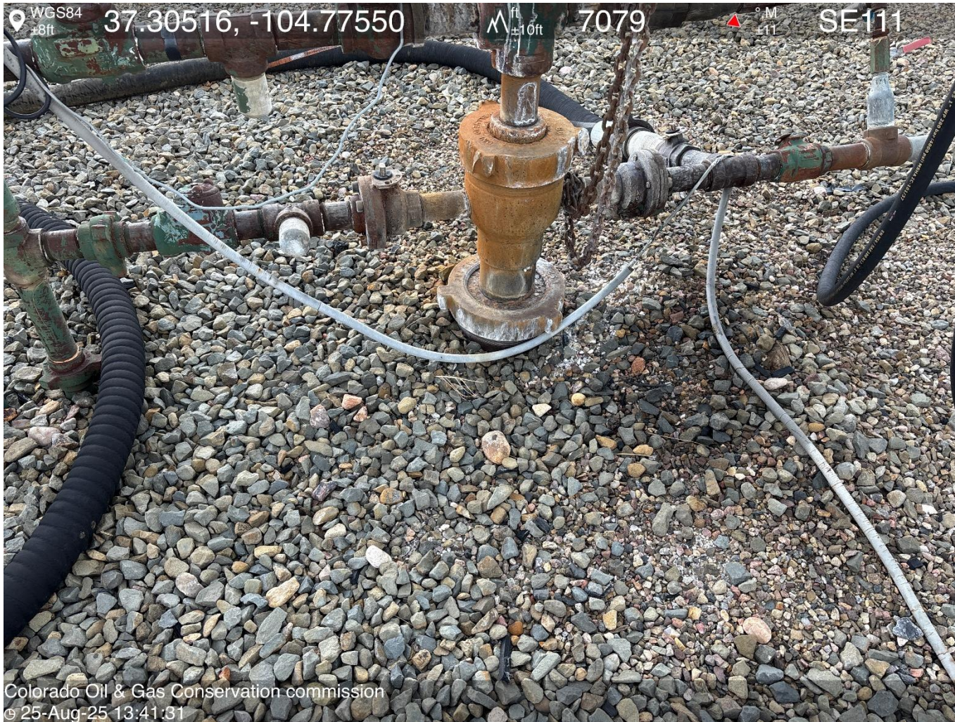
PHOTO 7: AREA OF IMPACTED SOIL NEAR WELLHEAD. Conduct maintenance on equipment, cleanup stained material and review self inspection processes. COMPLY WITH RULE 1002,(2).D. CA DATE 9-25-2025.
