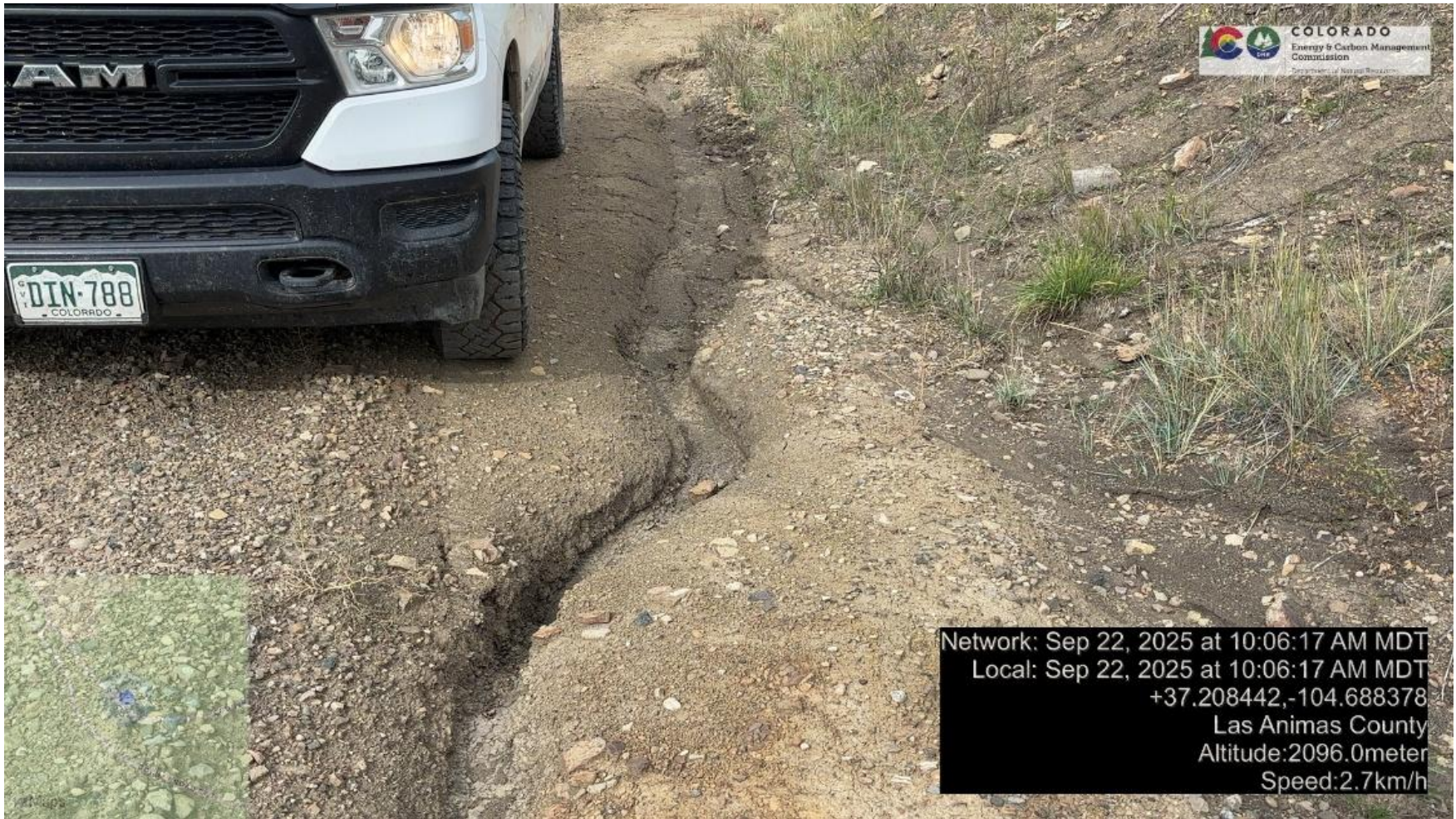
PHOTO 5: MORE EROSION ALONG ROW.
