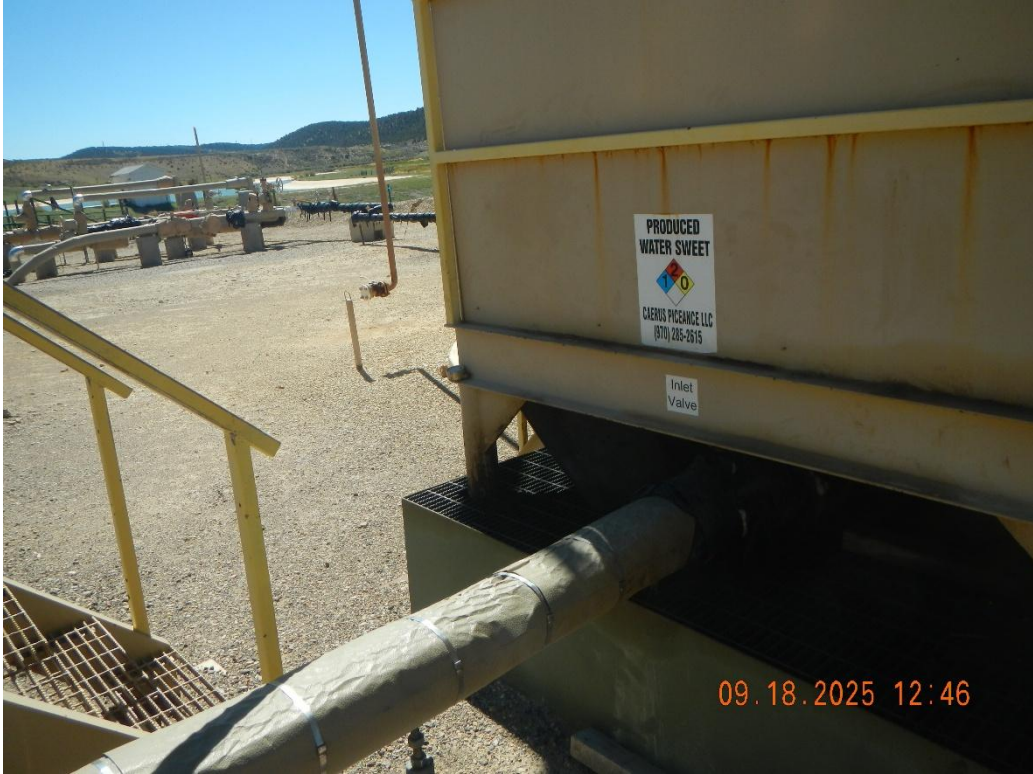
Filter station in tank berm.
