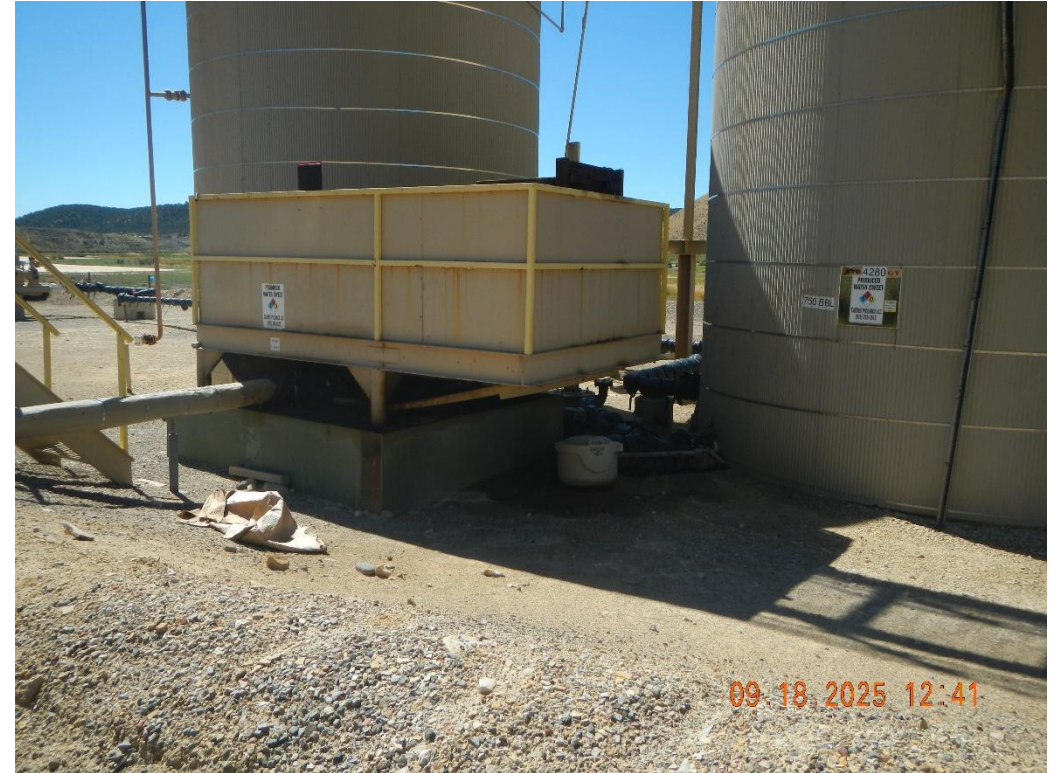
Filter station in tank berm.
