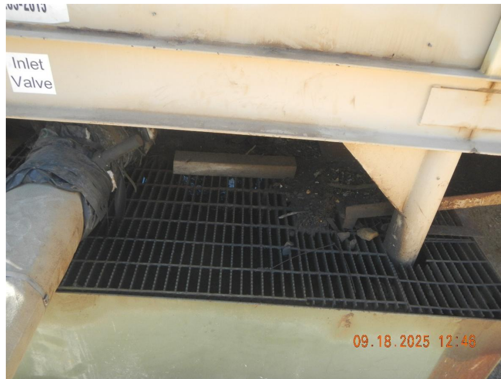
No walls above the grate and appears to allow spillage and built up debris on grate possibly causing fluids flow and/or splash out of catch tank.
