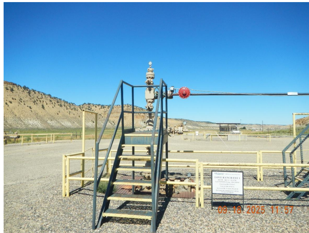
Metal tag on well line. No api#.
