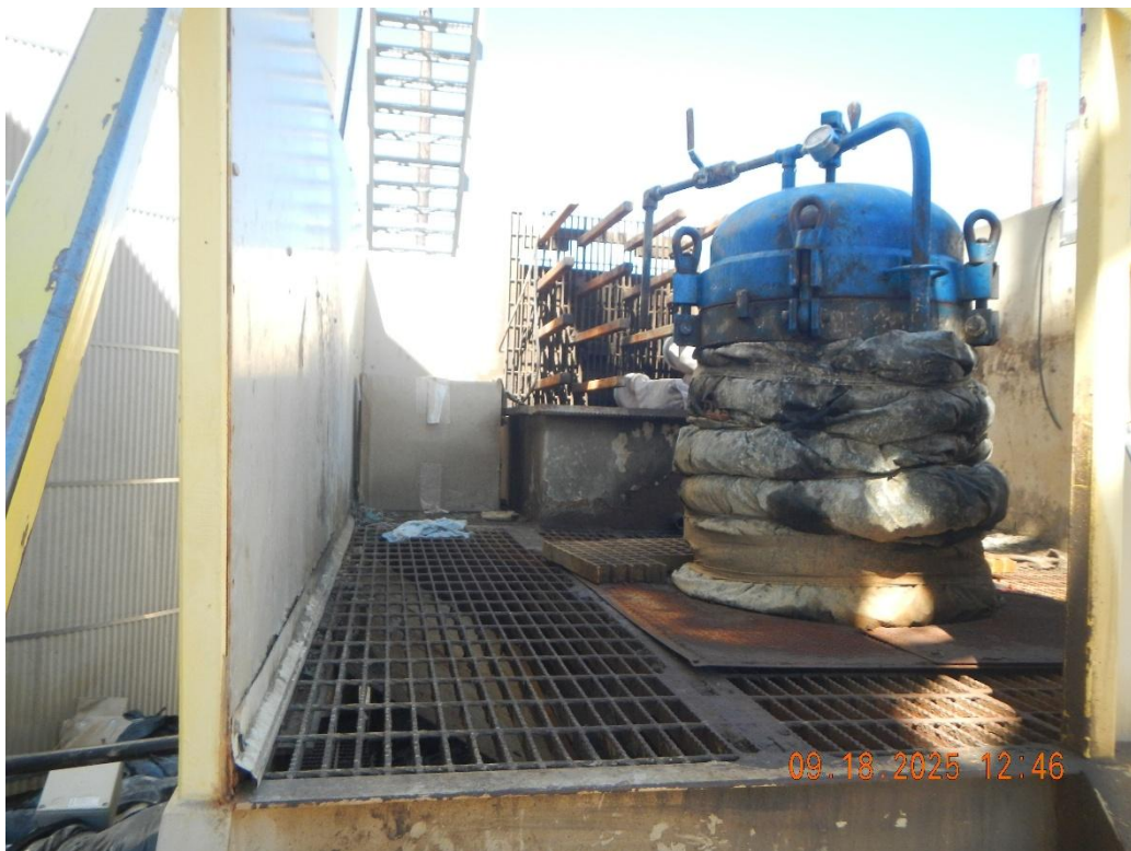
Filter station in tank berm.
