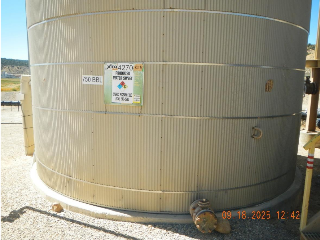
Product valve blocked.
