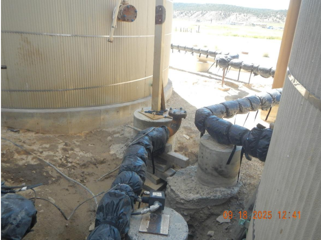
Line disconnected to production tank.
