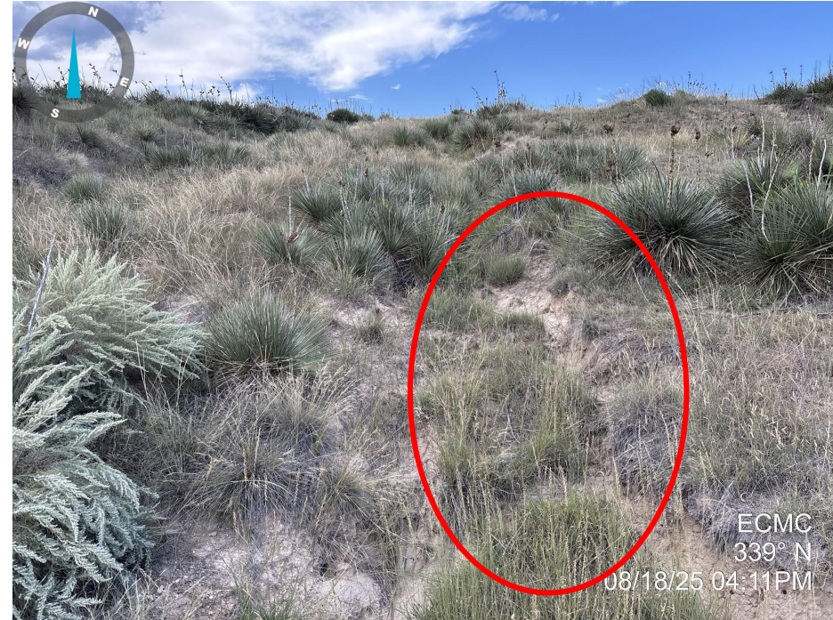
Photo 6. Photo taken of the access road to the well location, facing north, away from the location. Photo illustrates stormwater erosion, highlighted in red.
