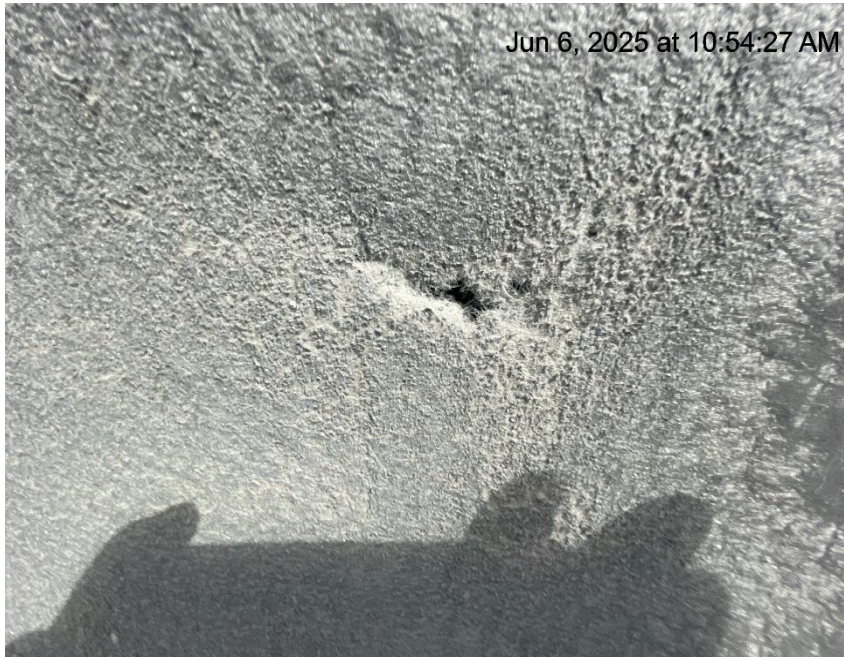
Photo # 6913 From inspection/audit 708906677 conducted on 06/06/2025 Hole in liner/liner needs maintenance
