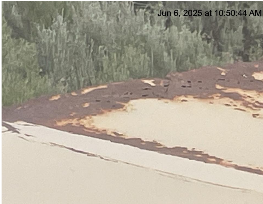
Photo # 6902 From inspection/audit 708906677 conducted on 06/06/2025 Tank failure Multiple holes in tank/tank lacks integrity
