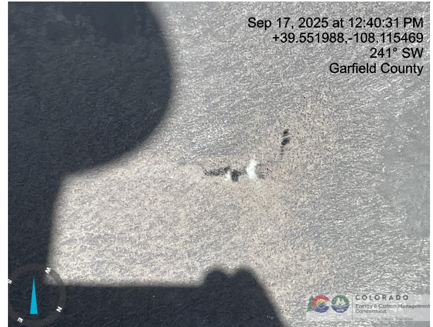
Photo # 290 Hole in liner/liner needs maintenance
