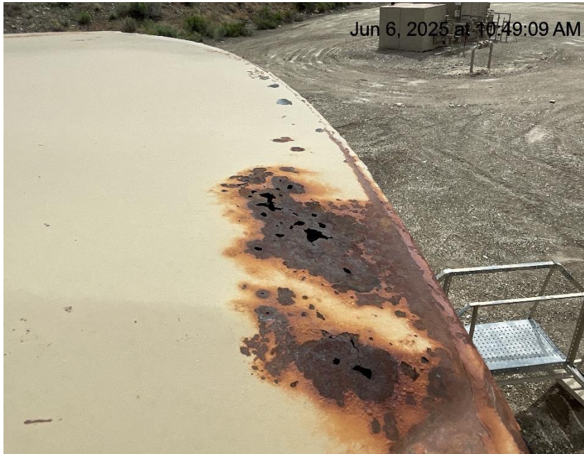
Photo # 6903 From inspection/audit 708906677 conducted on 06/06/2025 Tank failure Multiple holes in tank/tank lacks integrity
