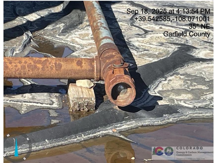
Photo # 1194 Open ended load line
