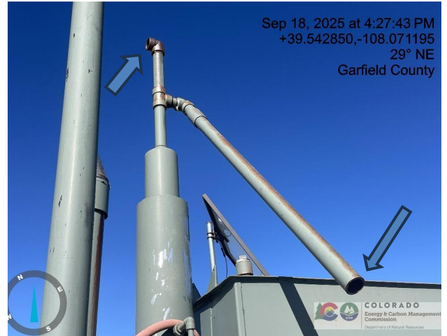
Photo # 1200 Open ended piping on separator/wildlife hazards/available for entry by wildlife
