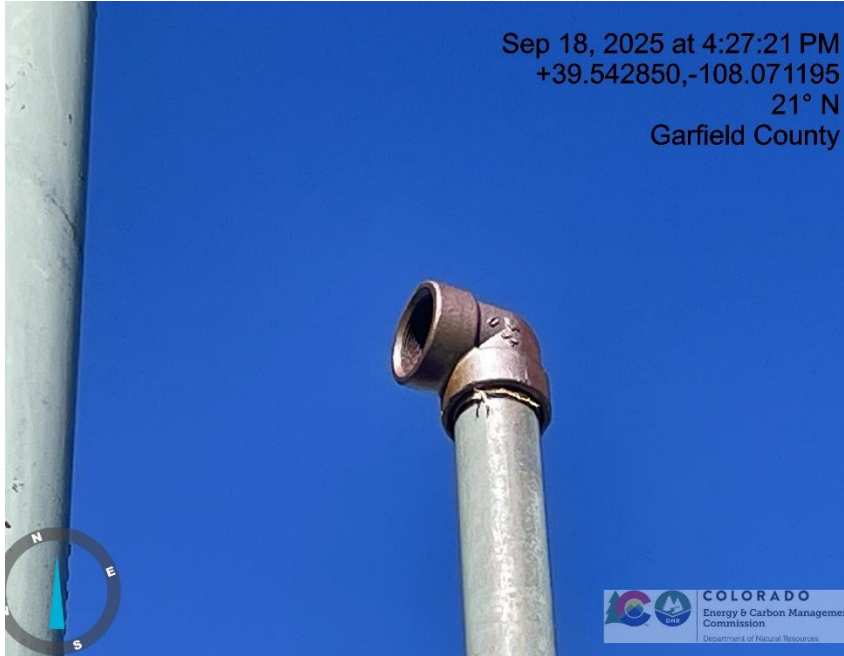
Photo # 1201 Open ended piping on separator/wildlife hazard/available for entry by wildlife
