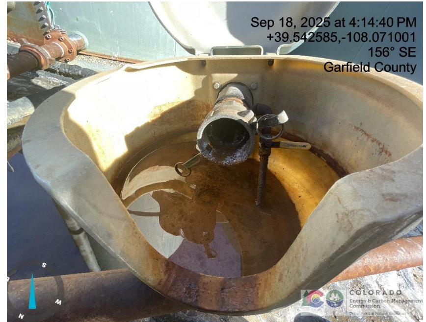
Photo # 1196 Open ended load line
