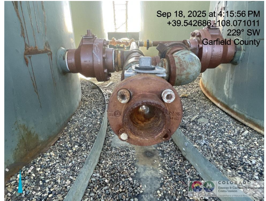
Photo # 1198 Open ended load line
