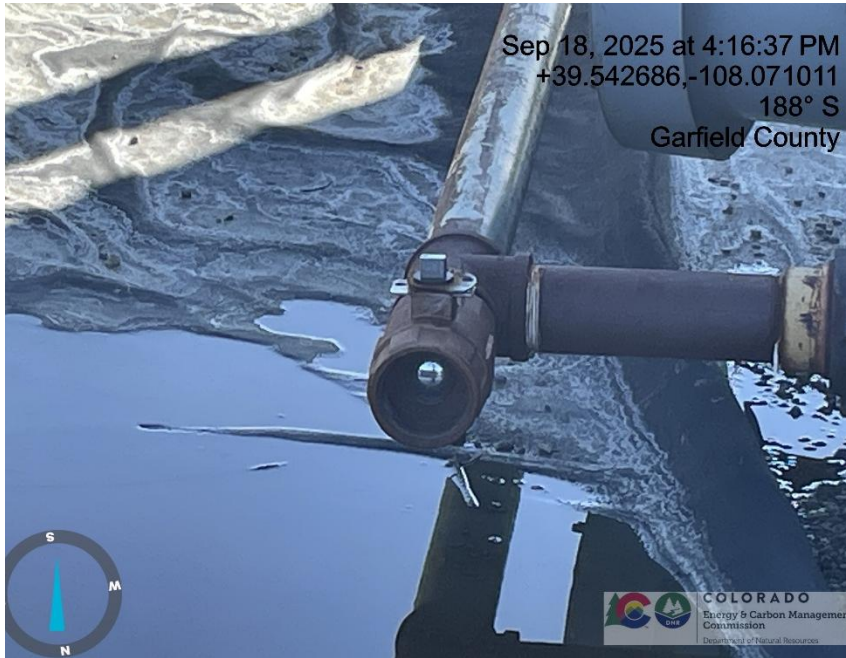
Photo # 1199 Open ended load line
