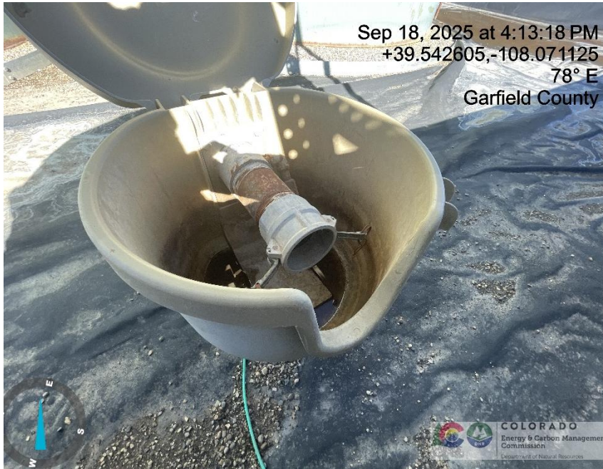
Photo # 1193 Open ended load line
