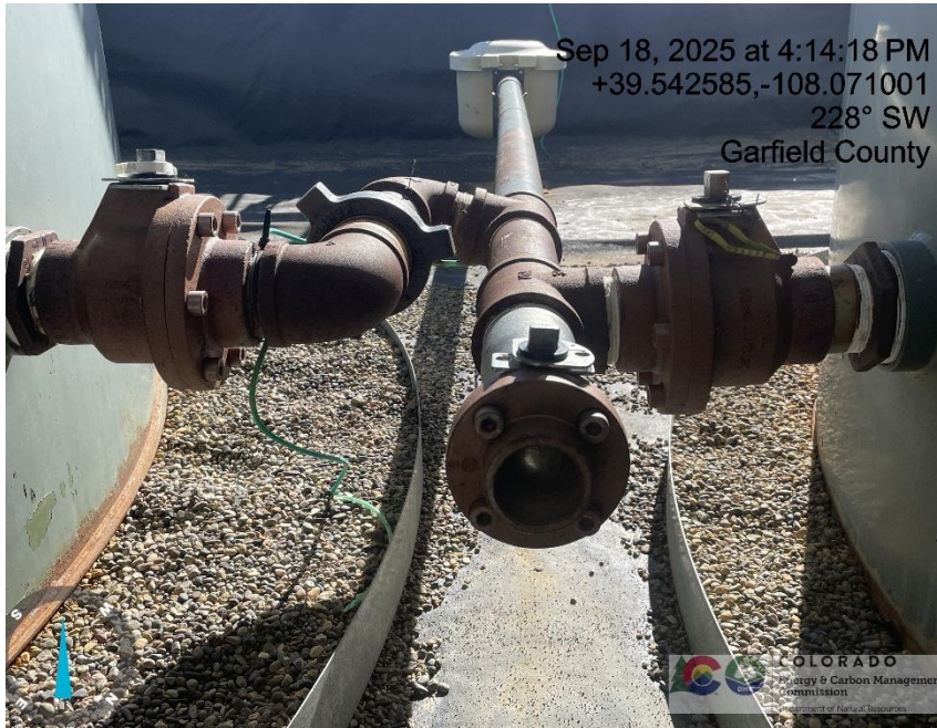
Photo # 1195 Open ended load line
