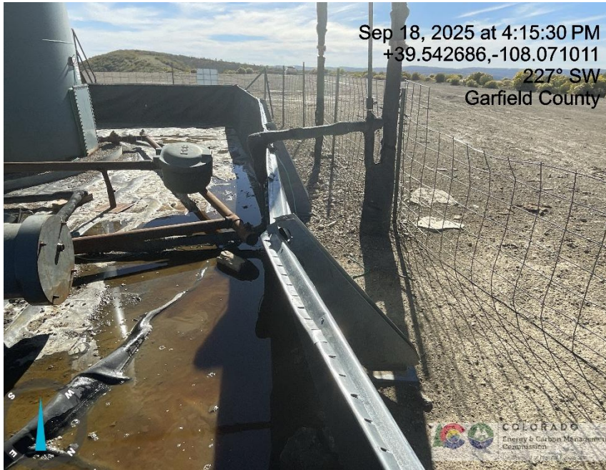
Photo # 1215 Tank battery containment showing some signs of damage
