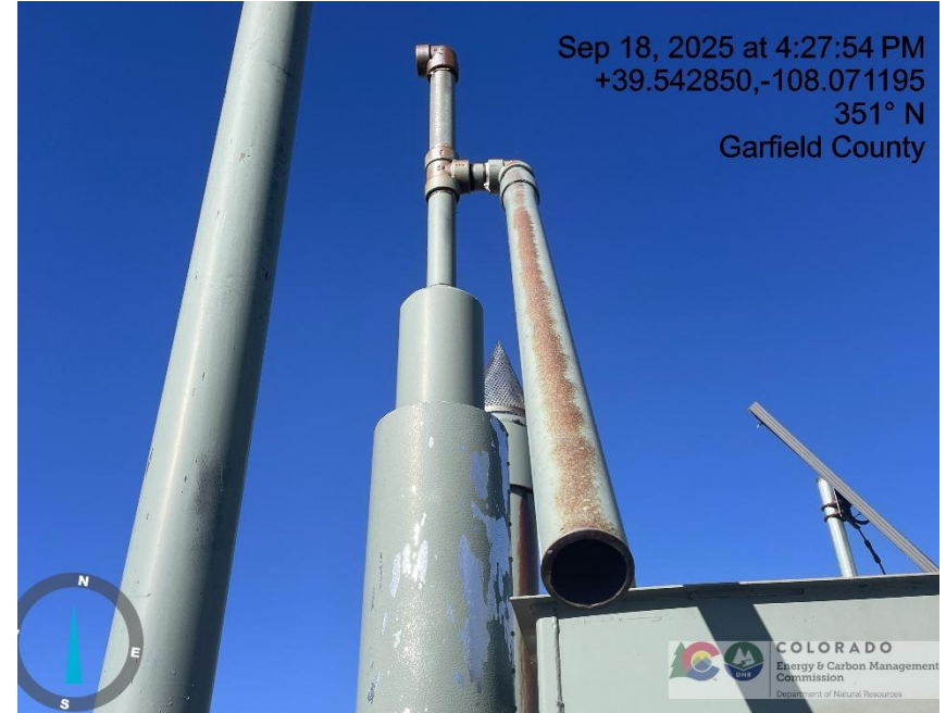
Photo # 1202 Open ended piping on separator/wildlife hazard/available for entry by wildlife
