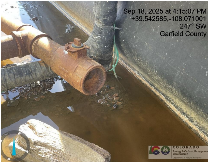
Photo # 1197 Open ended load line
