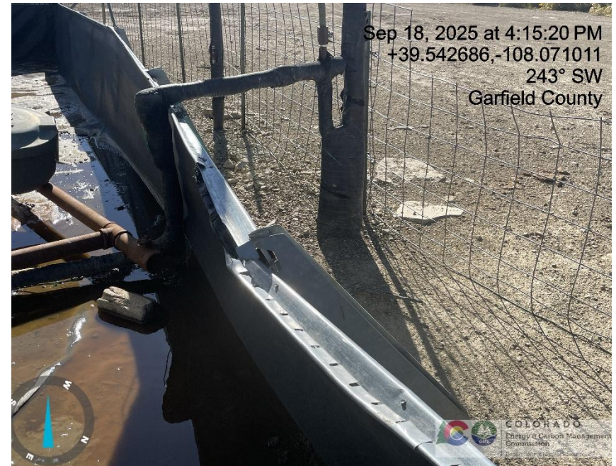
Photo # 1214 Tank battery containment showing some signs of damage
