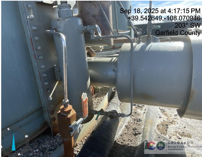
Photo # 1211 PRV vent line on tank burner does not comply with CECMC pressure safety device rules
