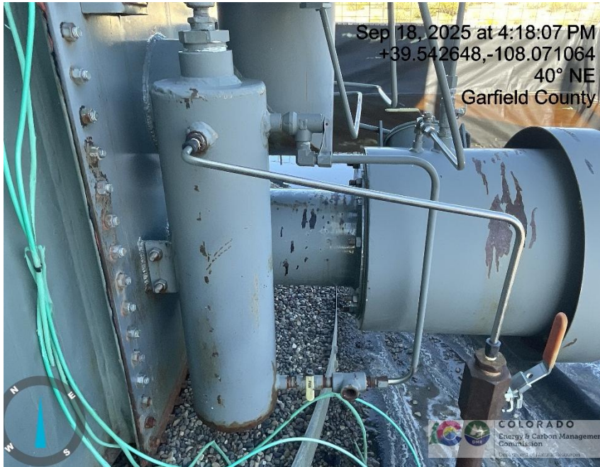
Photo # 1209 PRV vent line on tank burner does not comply with CECMC pressure safety device rules
