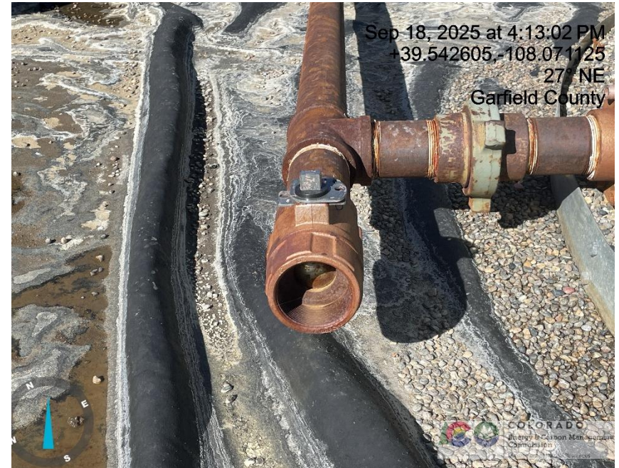
Photo # 1192 Open ended load line
