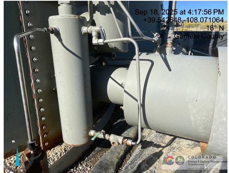
Photo # 1210 PRV vent line on tank burner does not comply with CECMC pressure safety device rules
