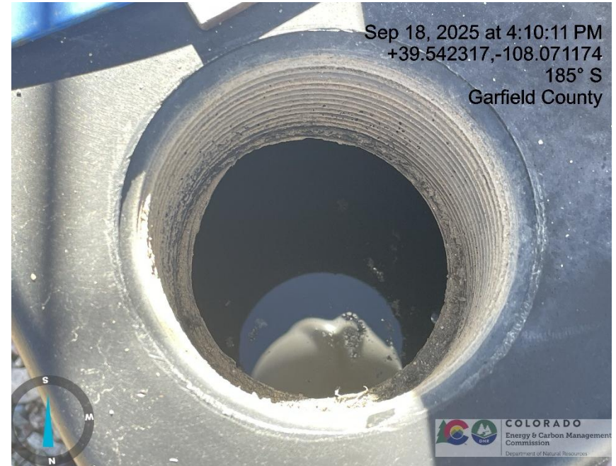
Photo # 1221 Failure to maintain chemical BMP/chemical tank containment approximately 3/4 to 7/8 full of fluid/BMP insufficient to contain possible spill
