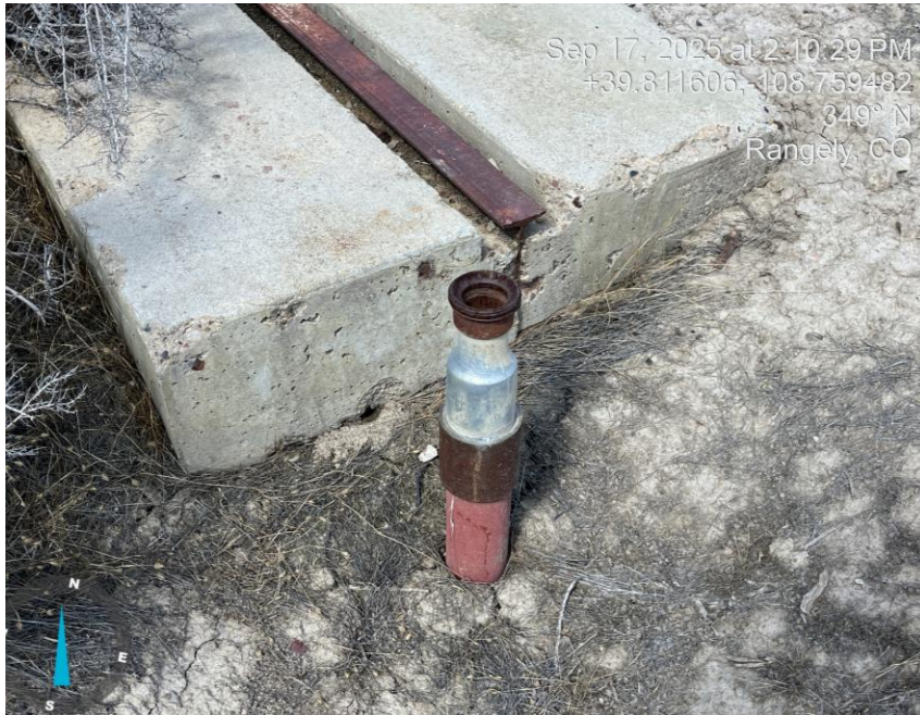
Photo # 3578 Open ended piping/wildlife hazard/available for entry by wildlife
