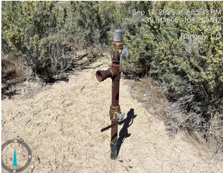
Photo # 3575 Unused flowline lacks lockout tagout (OOSLAT) & has open ended piping/wildlife hazard/available for entry by wildlife
