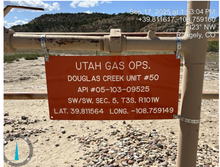
Photo # 3565 Wellhead sign lacks required information/not in compliance with CECMC rules
