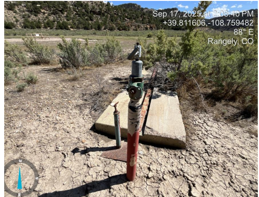
Photo # 3577 Unused flowline lacks lockout tagout (OOSLAT)
