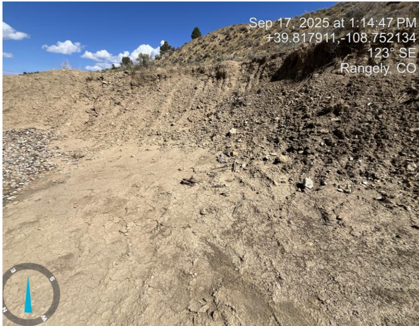
Photo # 3543 Erosion & transport of sediment on cutslope/sediment migrating onto location/insufficient BMP's
