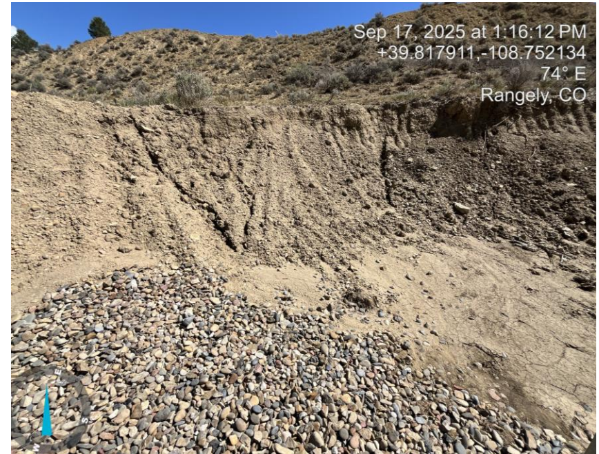
Photo # 3545 Erosion & transport of sediment on cutslope/sediment migrating onto location/insufficient BMP's
