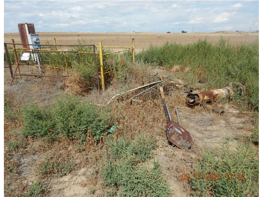
Unused equipment; electrical service Trash/ debris; well casing cut off and electrical/ pipe trash
